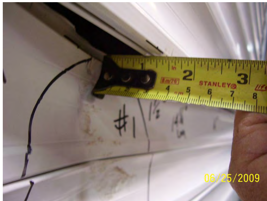
Photo No. 6 Specimen #2 after the Cyclic Pressure Test. An opening of 1" deep by 1/8" deep at each end by 14" long remained.
