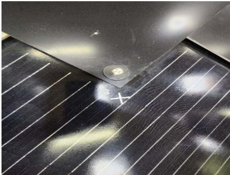
Photo No. 11 Impact Location #5 After Impact
