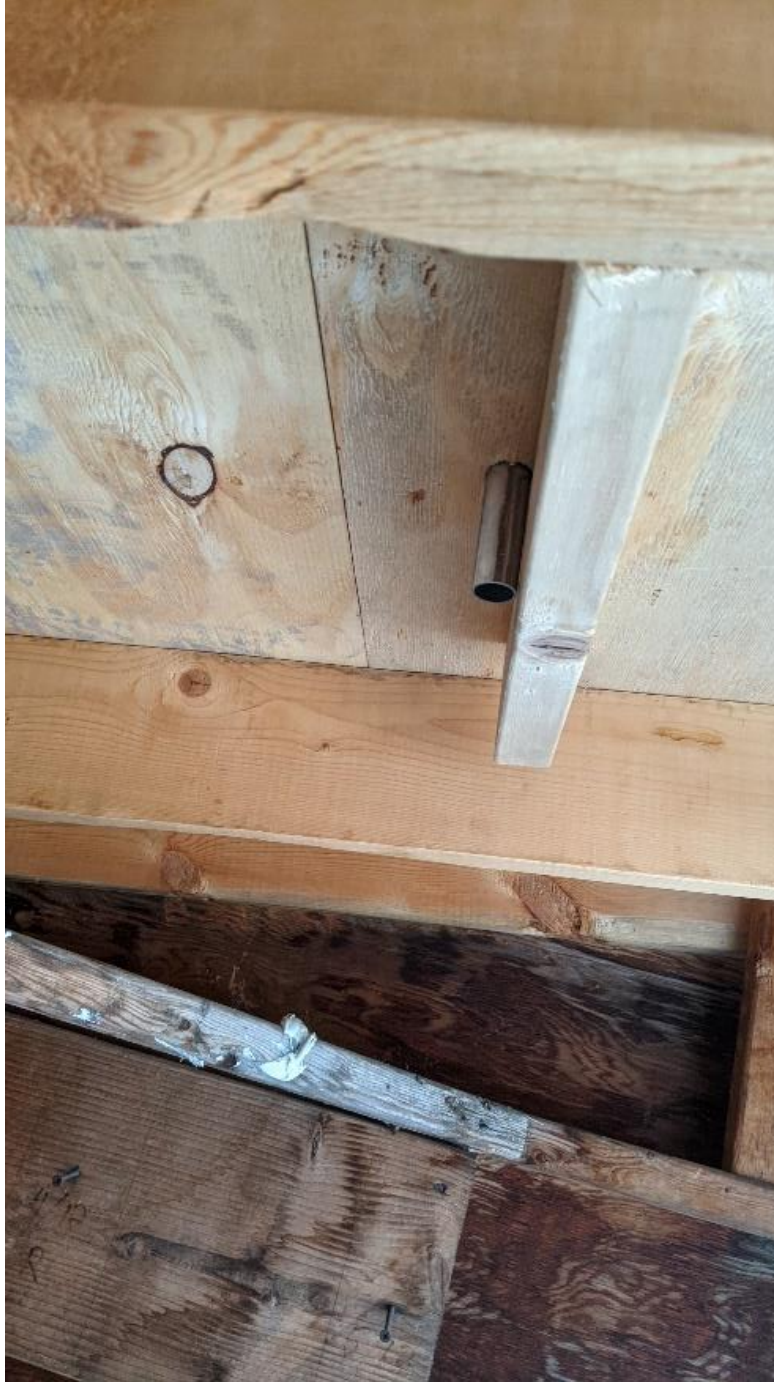
Photo No. 21 Post Test Underside
