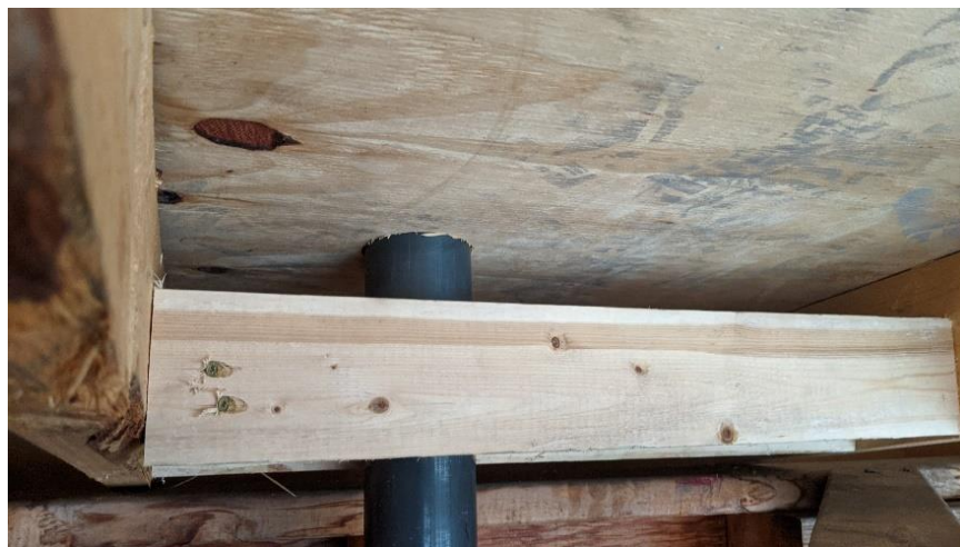
Photo No. 20 Post Test Underside
