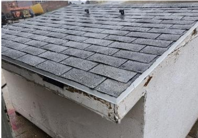
Photo No. 7 90 MPH Top side
