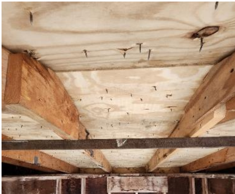
Photo No. 12 Post Test Underside
