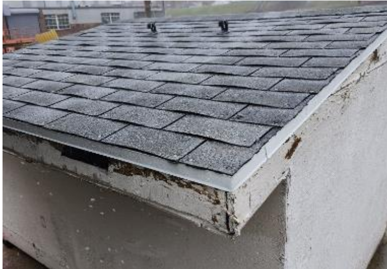
Photo No. 9 110 MPH Top Side
