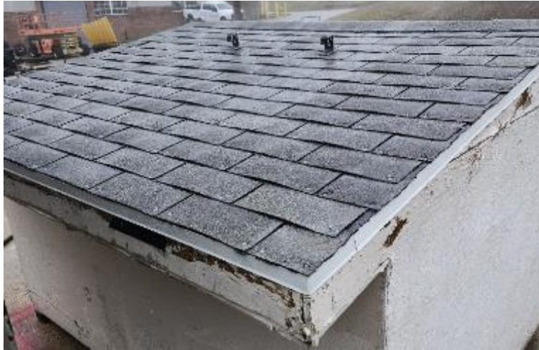
Photo No. 5 70 MPH Top Side
