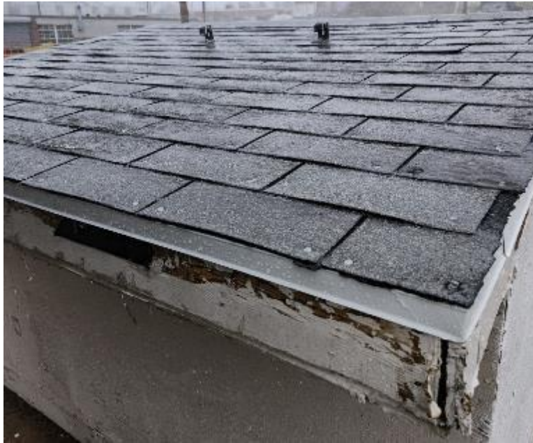
Photo No. 3 35 MPH Top Side
