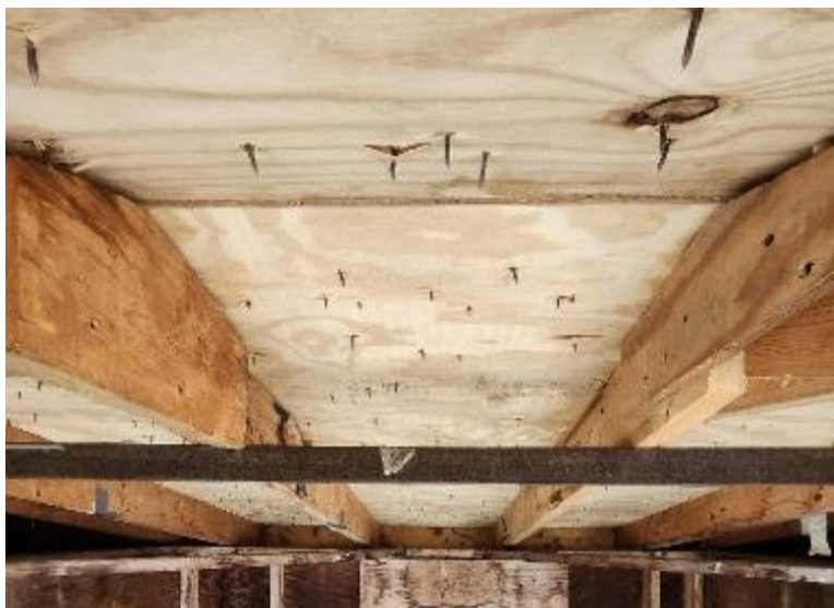
Photo No. 12 Post Test Underside
