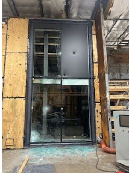
Photo No. 1 Talen Wall Impact
