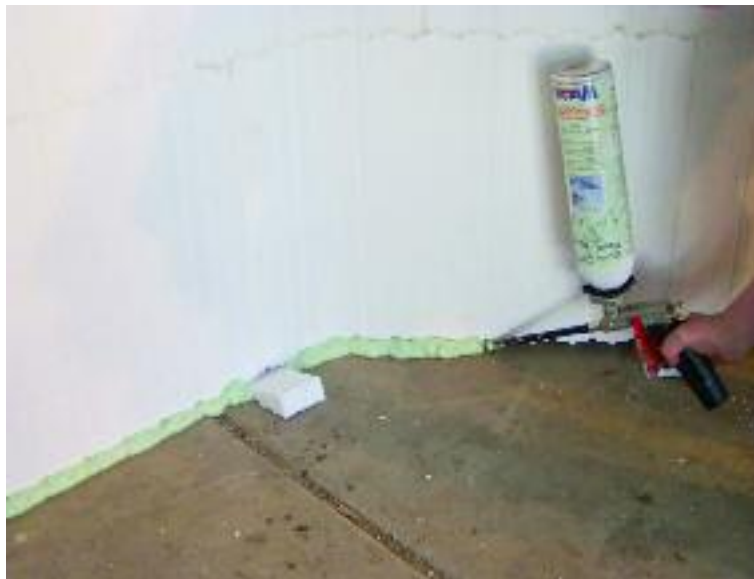
Figure 8.21 – Foaming under a large, low spot area
