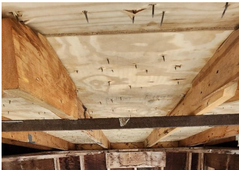
Photo No. 12 Post Test Underside
