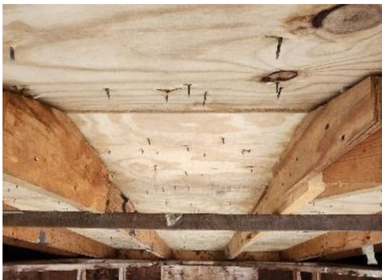
Photo No. 12 Post Test Underside
