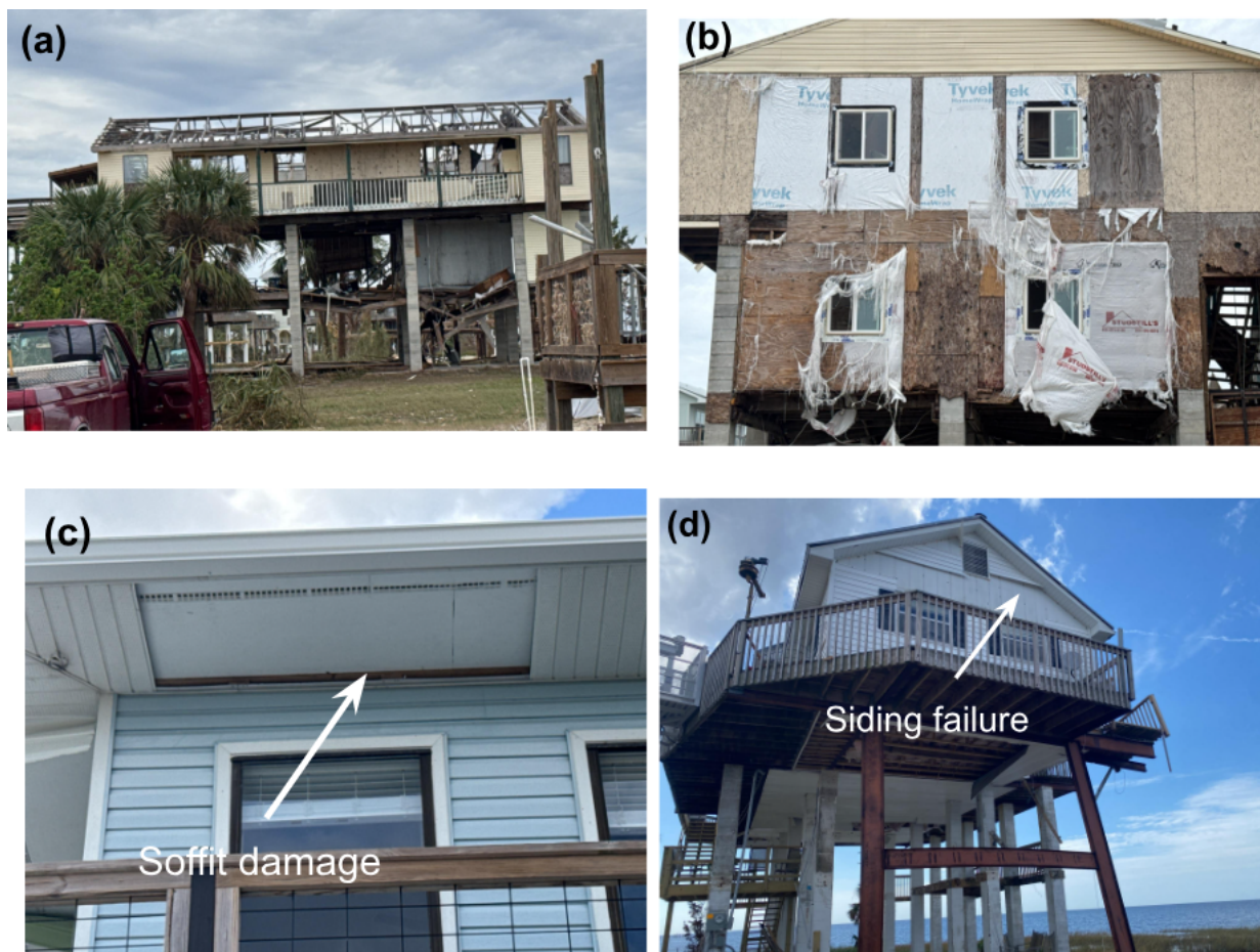
Figure 19. Examples of poor wind performance in buildings within the affected community: (a) a one-story home on Dekle Beach Blvd, built in 1998 on 16-foot elevated reinforced masonry piers , experienced roof structure and sheathing failure. The home featured an 8-foot elevated deck extending over the entire floor plan, which, along with part of it enclosed by wood framed walls the living area built on it, likely failed due to surge and wave loading; (b) siding damage observed on the same home; (c) soffit partially removed along the eave of a house constructed in 1983, Dekle Beach and (d) vinyl siding that was installed over existing wood siding system of house (originally constructed in 1945) was partially stripped from the northeast elevation (i.e., gable end) siding damage on elevated buildings located in Dekle Beach, constructed in 1983 and 1945 , respectively.
