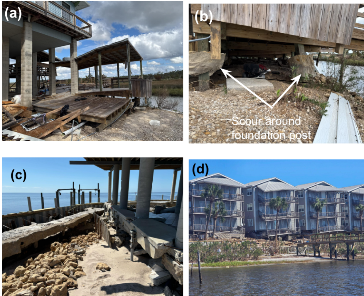
Figure 16. Examples of uplift, scour, and erosion effects on coastal buildings during Hurricane Helene: (a) uplift of a slab-on-grade floor deck and (b) scour around the post foundation of a single-family home in Dekle Beach built in 1983; (c) erosion and scour affecting the open ground story floor slab and waterfront of a single-family home built in 1980 in Horseshoe Beach; and (d) scour and erosion around the foundation of multi-story Seashore Landing Condominiums in Cedar Key, constructed in 1995.
