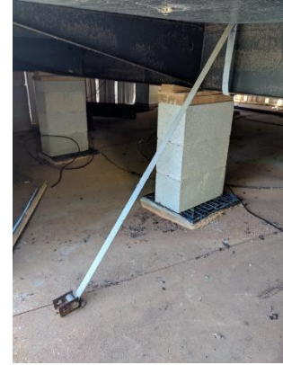
Ground anchors and strapping
