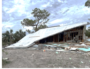
(b) Partially collapsed
