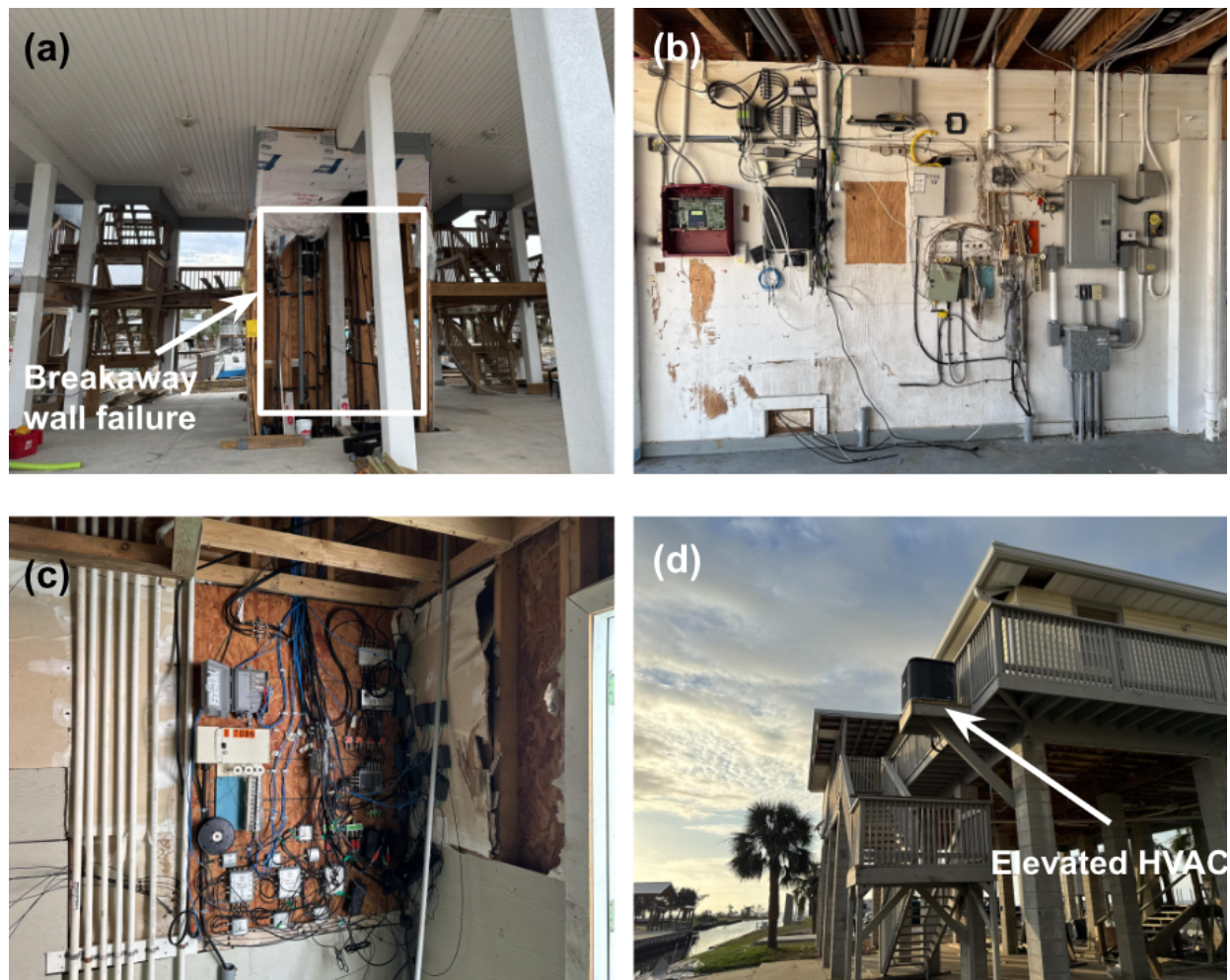
Figure 20. Performance of breakaway walls and utilities during Hurricane Helene: (a) designed failure of breakaway walls exposing the elevator shaft in a multi-story condominium on Keaton Beach Rd, built in 2005; (b) water damage to utilities in the open ground story of a multi-story condominium built in 2007, north of the Steinhatchee Marina; (c) enclosed utilities in the ground story of a multi-story condominium south of the Steinhatchee Marina; and (d) an elevated air-conditioning unit elevated to 13 ft above ground in Horseshoe Beach home built in 1995 that remained undamaged.
