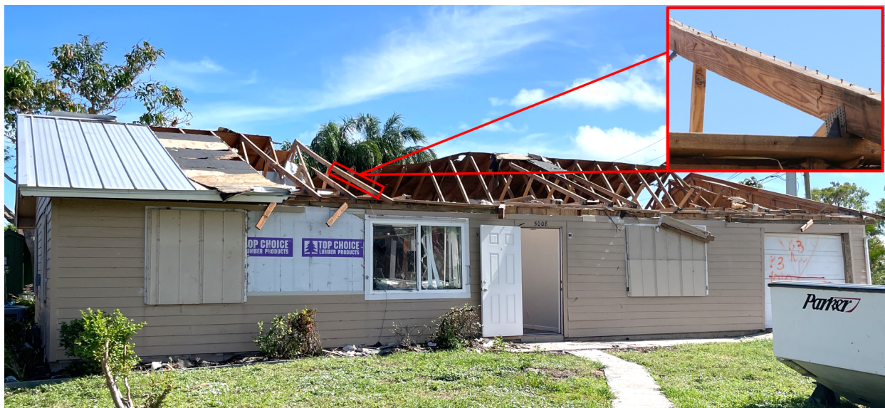
Figure 32. Severe structural roof damage to a wood-frame home constructed in 1977 that was retrofitted in 2017 and 2020 to install impact-rated windows, re-nail plywood roof deck, and install a metal roof. The inset shows a typical roof truss top chord with fasteners all remaining embedded in the truss, with failure of the roof deck due to fastener pull-through.
