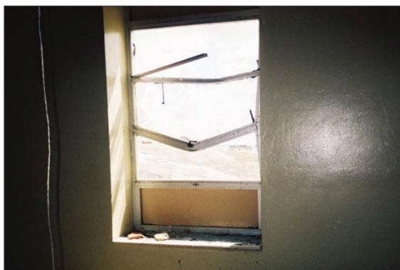
Figure 21. Broken window caused by wind-borne debris in a high school in Punta Gorda during Hurricane Charley (2004).
