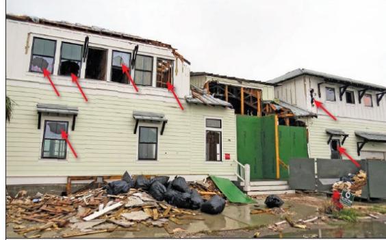
Figure 27. Damage in a post-2009 home caused by the impact of wind-borne debris (red arrows) in a Key Allegro house during Hurricane Harvey (2017). EWS = 140 mph, exposure C.
