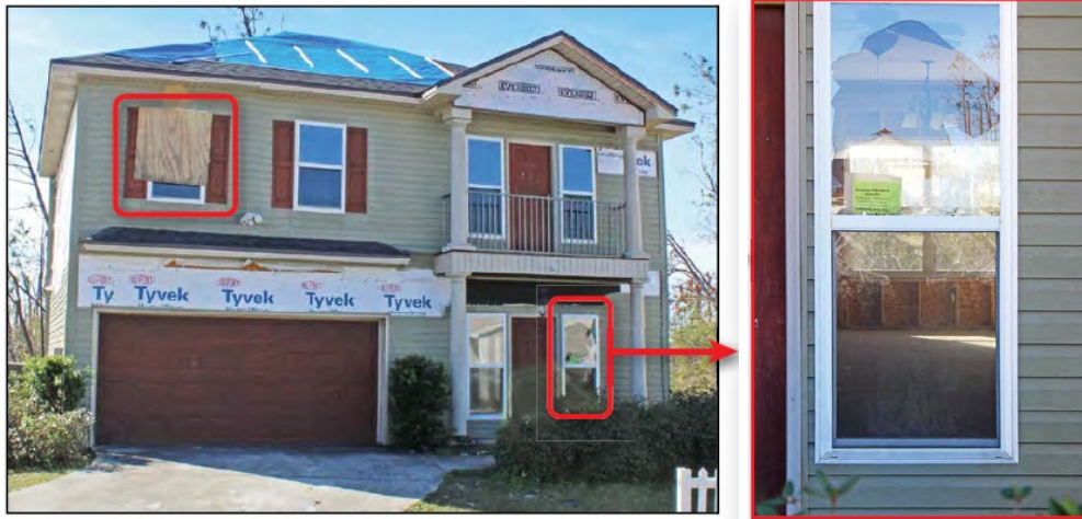
Figure 41. Glazed opening damage after Hurricane Michael (2018) in a house built in 2005, located in Panama City. Estimated wind speeds (128 mph) approached the design wind speed (133 mph).
