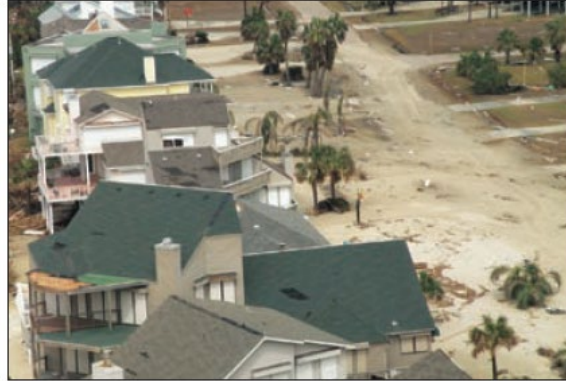
Figure 22. Siding and roofing materials blew off these West Galveston houses during hurricane Ike (2008) becoming potential projectiles.
