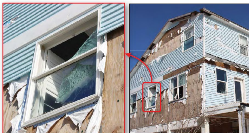
Figure 40. Impact resistant window after Hurricane Michael (2018) in a house built in 2010, located in Mexico Beach. Estimated wind speeds (150 mph) exceeded the design wind speeds (130 mph).
