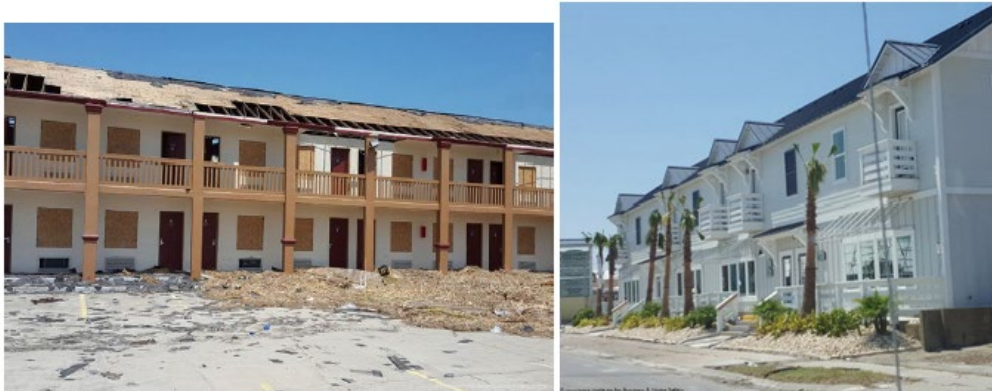
Figure 36. Port Aransas North: Two commercial buildings located 1 mile apart that experienced similar wind speeds during hurricane Harvey (2017). 1984 construction (left), 2007 construction (right).
