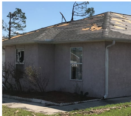
Figure 48. Damage to windows in a house located in Panama City during Hurricane Michael (2018). House was built between 1990-1999 and located 3.25 miles from St. Andrew Bay. Estimated wind speeds (129-150 mph) might have exceeded the design wind speeds (135 mph).
