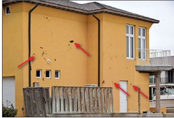
Figure 30. Damage on stucco walls (red arrows) caused by small debris impact in Key Allegro. EWS = 120 mph, exposure C.
