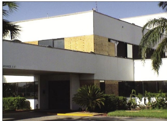
Figure 12. Damage in the windows in a hospital in Arcadia during Hurricane Charley (2004). EWS = 110-120 mph.
