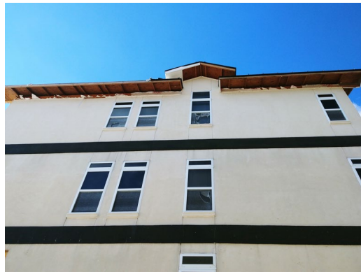
Figure 50. Damage to a few windows in the shoreline of Mexico Beach during Hurricane Michael (2018). House was built between 2000-2009. Estimated wind speeds (150 mph) exceeded the design wind speeds (136 mph).
