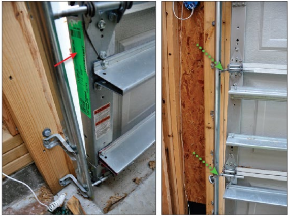
Figure 26. Damage caused by debris impact resulting in two bent rollers in Fulton during Hurricane Harvey (2017). EWS = 130 mph, exposure B.
