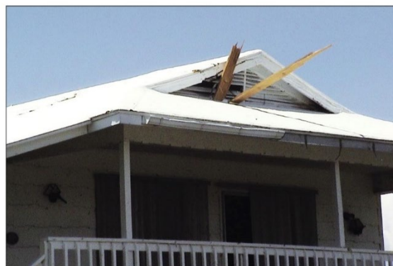
Figure 10. Impact of structural wood in the gable end in Pine Island during Hurricane Charley (2004)
