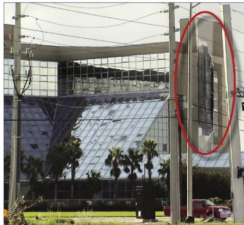
Figure 7. Damage to glass atrium in Orlando caused by wind-borne debris during Hurricane Charley (2004).
