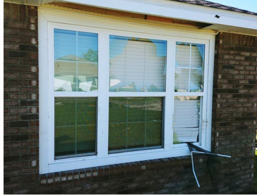
Figure 49. Damage to a window in Panama City during Hurricane Michael (2018). House was built between 2010-2019 and located 3.39 miles from St. Andrew Bay. Estimated wind speeds (129-150 mph) might have exceeded the design wind speeds (135 mph).
