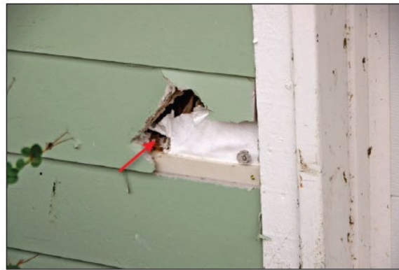
Figure 28. Damage on fiber cement siding (red arrow) caused by the impact of wind-borne debris in a Key Allegro house during Hurricane Harvey (2017). EWS = 120 mph, exposure C.
