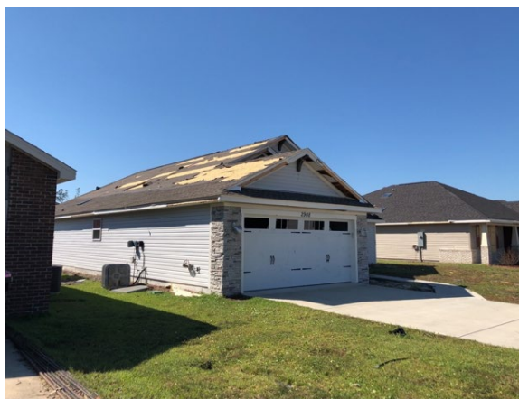
Figure 46. Damage to roof and garage door in Panama City during Hurricane Michael (2018). House was built between 2000-2009 and located 3.39 miles from St. Andrew Bay. Estimated wind speeds (129-150 mph) might have exceeded the design wind speeds (135 mph).
