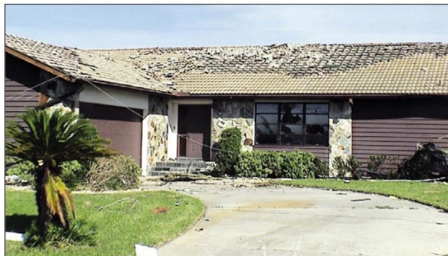
Figure 5. Extensive damage of pre-2001 FBC home. Broken windows caused by wind-borne debris during Hurricane Charley (2004).
