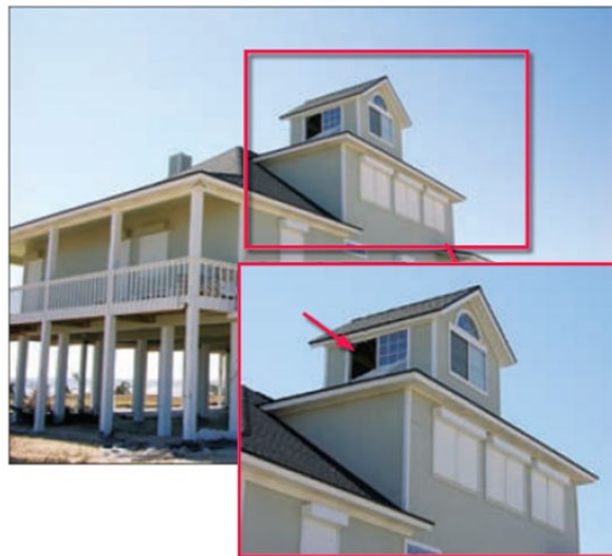
Figure 23. Window vulnerable to wind-borne damage due to improper installation of shutters.
