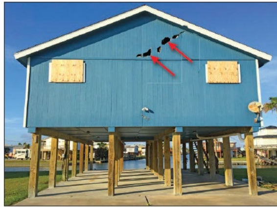
Figure 31. Damage on hardboard siding (red arrow) caused by multiple impact of debris in a Holiday Beach house during Hurricane Harvey (2017). EWS = 120 mph, exposure C.
