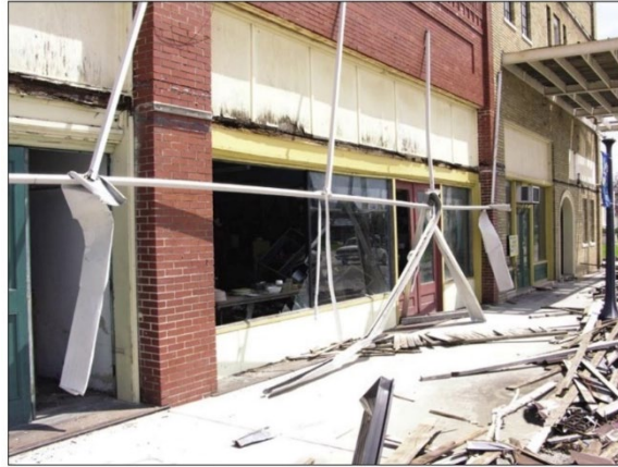
Figure 19. Broken glass windows caused by wind-borne debris during hurricane Charley (2004) in Wauchula.
