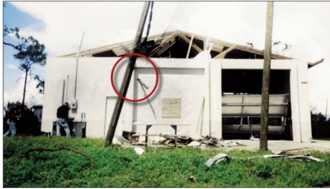
Figure 13. Fire station with a missile (in the red circle) caused by Hurricane Charley (2004), in Punta Gorda.
