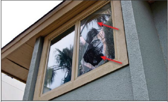
Figure 25. Damage in a window caused by the impact of wind-borne in a Key Allegro house during Hurricane Harvey (2017).
