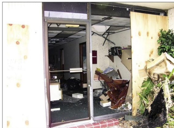
Figure 15. Broken windows in an office caused by Hurricane Charley (2004) in Punta Gorda.
