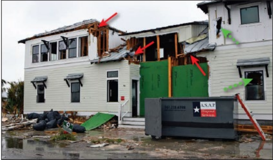
Figure 24. Damage caused by wind-borne debris (green arrows) and wind uplift damage (red arrows) in a house in Rockport during Hurricane Harvey (2017). EWS = 130 mph, exposure C.
