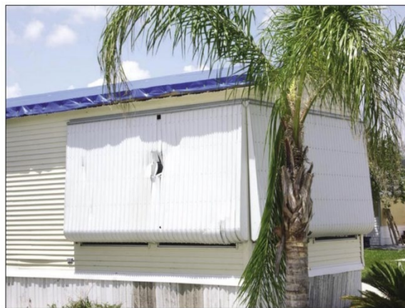
Figure 18. Metal awning shutter penetrated by a missile in Zolfo Springs during hurricane Charley (2004).
