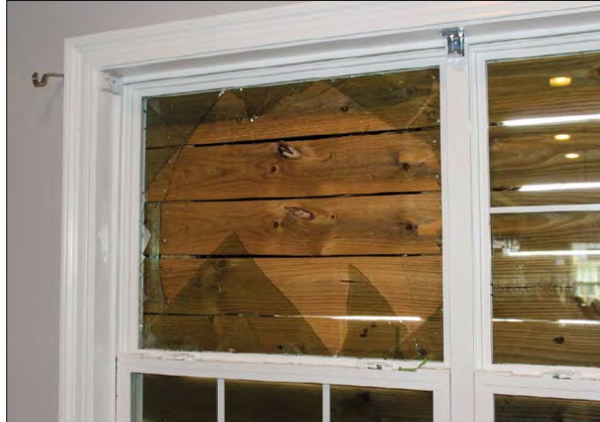
Figure 43. Glazed opening damage caused by an asphalt shingle after Hurricane Michael (2018) in a house built in 2012, located in Panama City. Estimated wind speeds (150 mph) exceeded the design wind speeds (126 mph).
