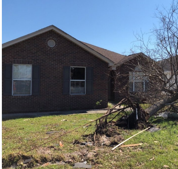
Figure 47. Damage to a window cause by wind-borne debris in Panama City during Hurricane Michael (2018). House was built between 2000-2009 and located 3.27 miles from St. Andrew Bay. Estimated wind speeds (129-150 mph) might have exceeded the design wind speeds (135 mph).
