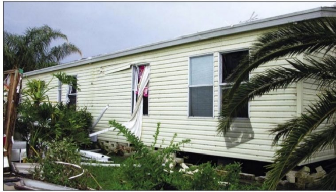
Figure 16. Windows broken in a manufactured home by wind-borne debris during Hurricane Charley (2004) at the east of Port Charlotte.
