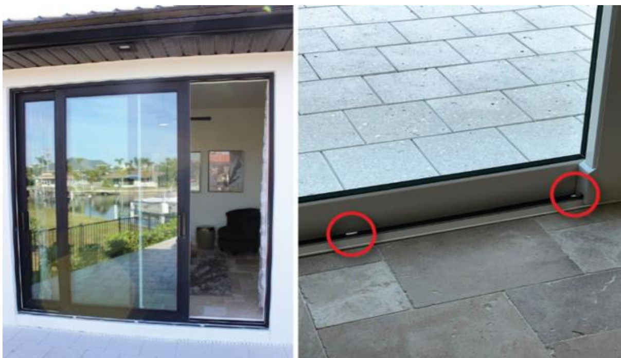
Figure 2 Due to WDR, a 2021 home with a two-panel SGD suffered severe water intrusion (the two red circles indicate weep holes that allow water to depart). DWS is 11 mph, and EWS is 130 mph. (Punta Gorda)
