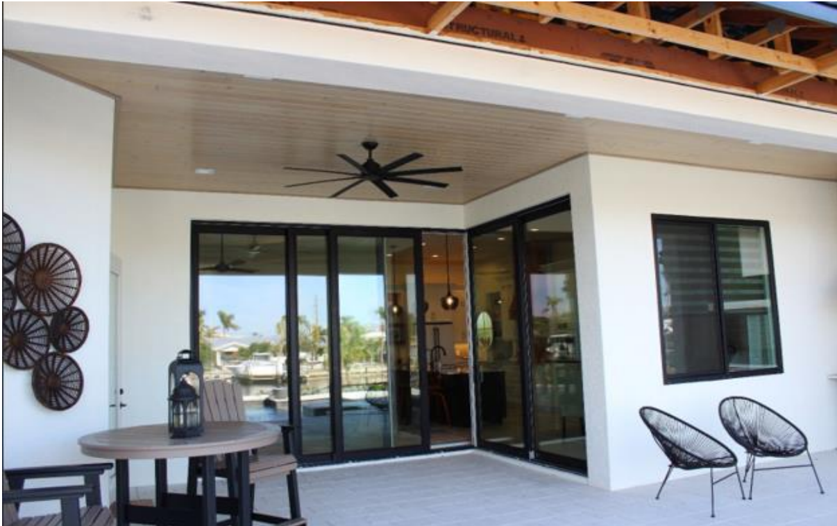
Figure 1: Significant water intrusion occurred in a 2021-built home with two and three panel SGD's (EWS = 130 mph; DWS = 151 mph) (Punta Gorda)
