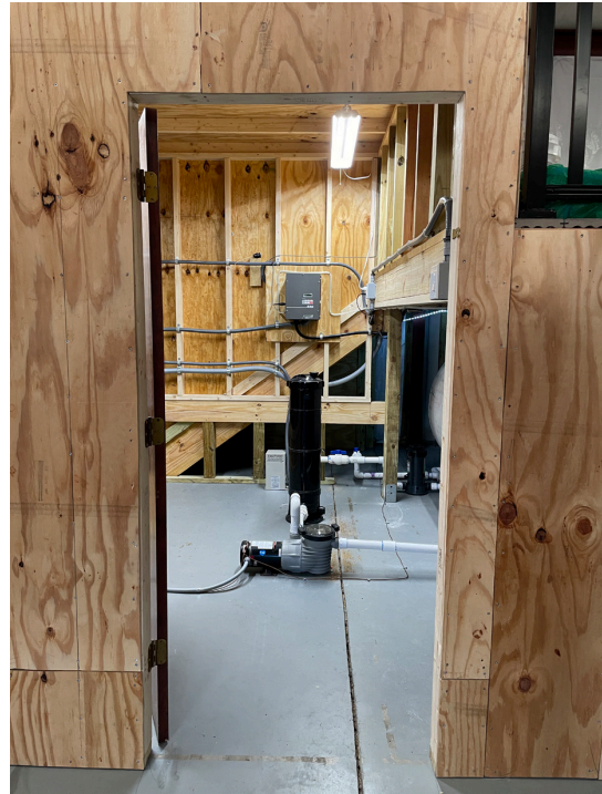
View through door into pump room
