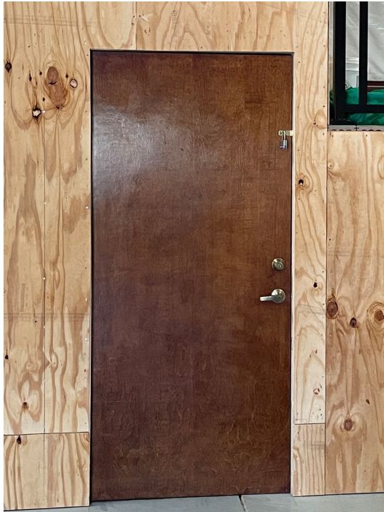
Entry door to pump room and pool access
