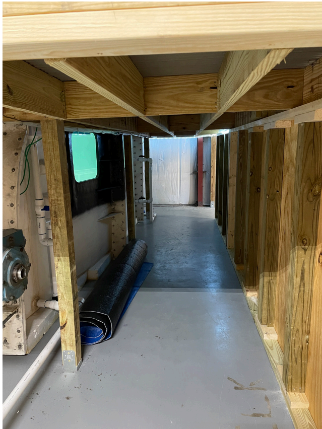
View down exterior deck wall from pump room
