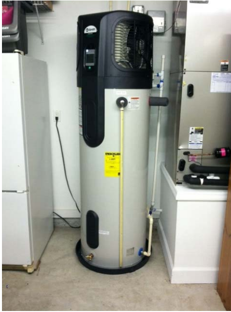
Figure 1 Heat pump water heater saved 70% of water heating energy use when it replaced electric resistance unit at "site #8" of recent DOE/FPL funded retrofit study
