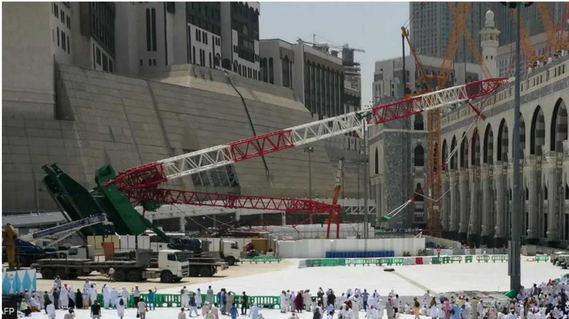
Figure 4-1. Fallen crawler crane at the Great Mosque in Saudi Arabia (AFP).
