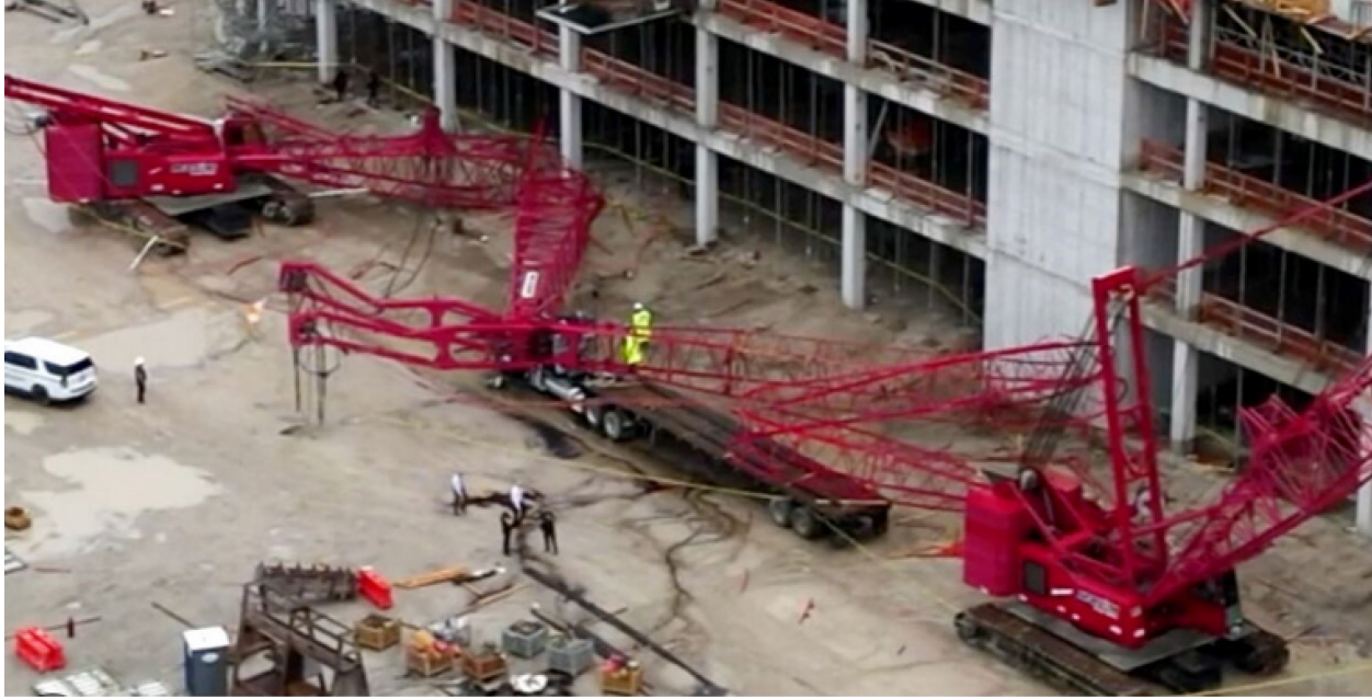
Figure 4-4. Collapsed crawler crane while constructing a hospital in Merritt Island. [17]
