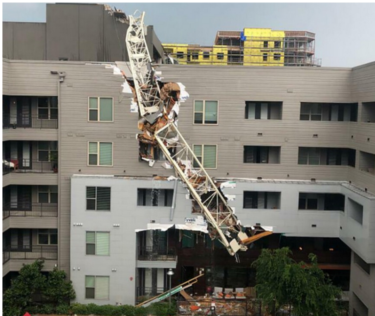
Figure 4-8. Tower crane that collapsed into a building in Dallas, Texas. (Michael Santana/AP)
