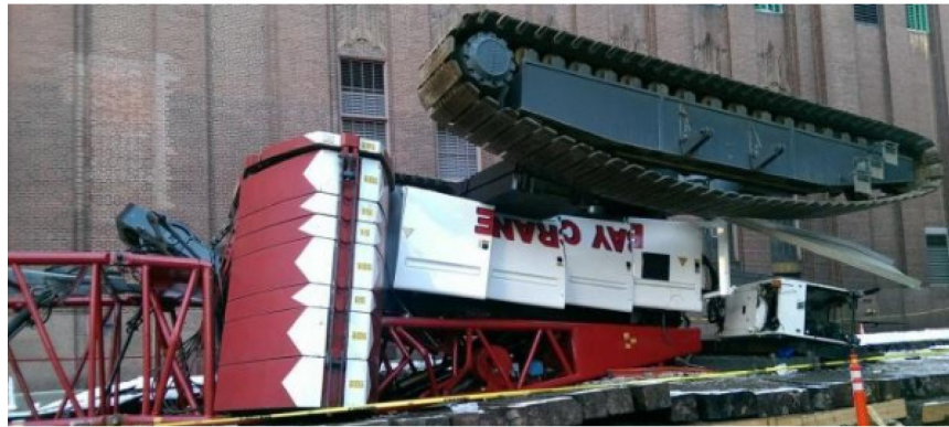
Figure 4-3. Overturned crawler crane in New York City. [16]
