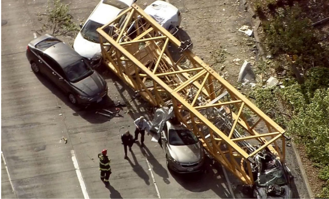
Figure 4-11. Crane failure in Seattle, Washington. (KIRO7.com)
