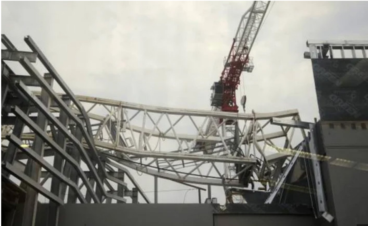
Figure 4-10. Crane failure in Richardson, Texas. (Meg Roussos / The Dallas Morning News)
