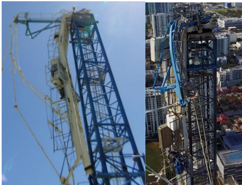
Figure 4-7. One example of the failed cranes in South Florida during Hurricane Irma. [21]
