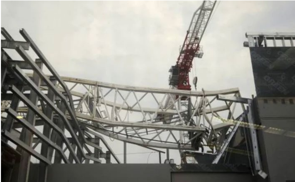
Figure 5-10. Crane failure in Richardson, Texas. (Meg Roussos / The Dallas Morning News)
