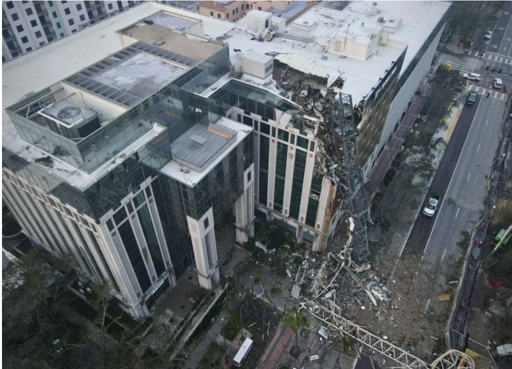
Figure 5-9. Tower crane collapsed into building in St. Petersburg, Florida. [25]
