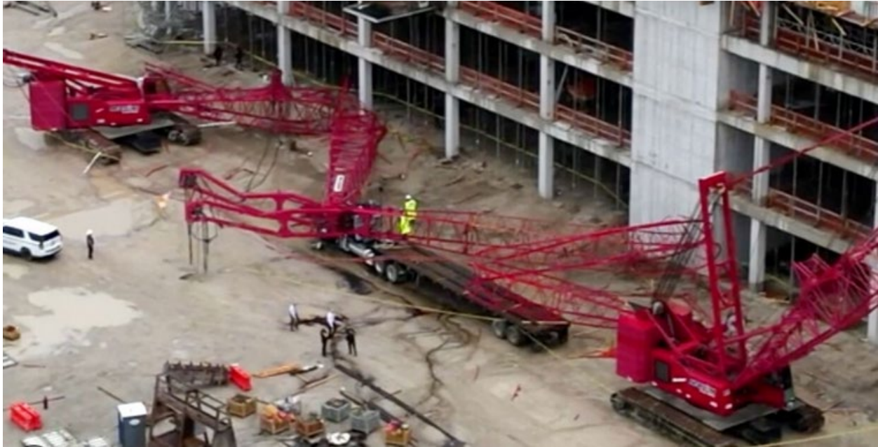
Figure 5-4. Collapsed crawler crane while constructing a hospital in Merritt Island. [17]
