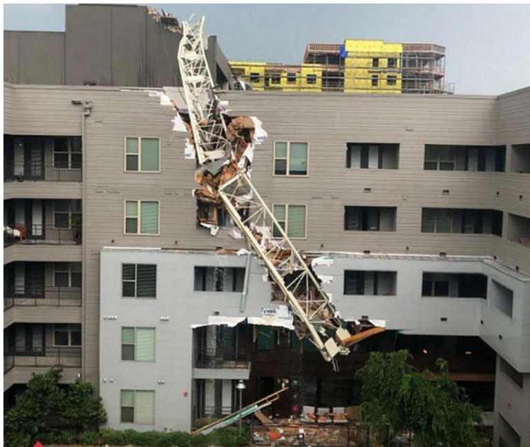
Figure 5-8. Tower crane that collapsed into a building in Dallas, Texas. (Michael Santana/AP)
