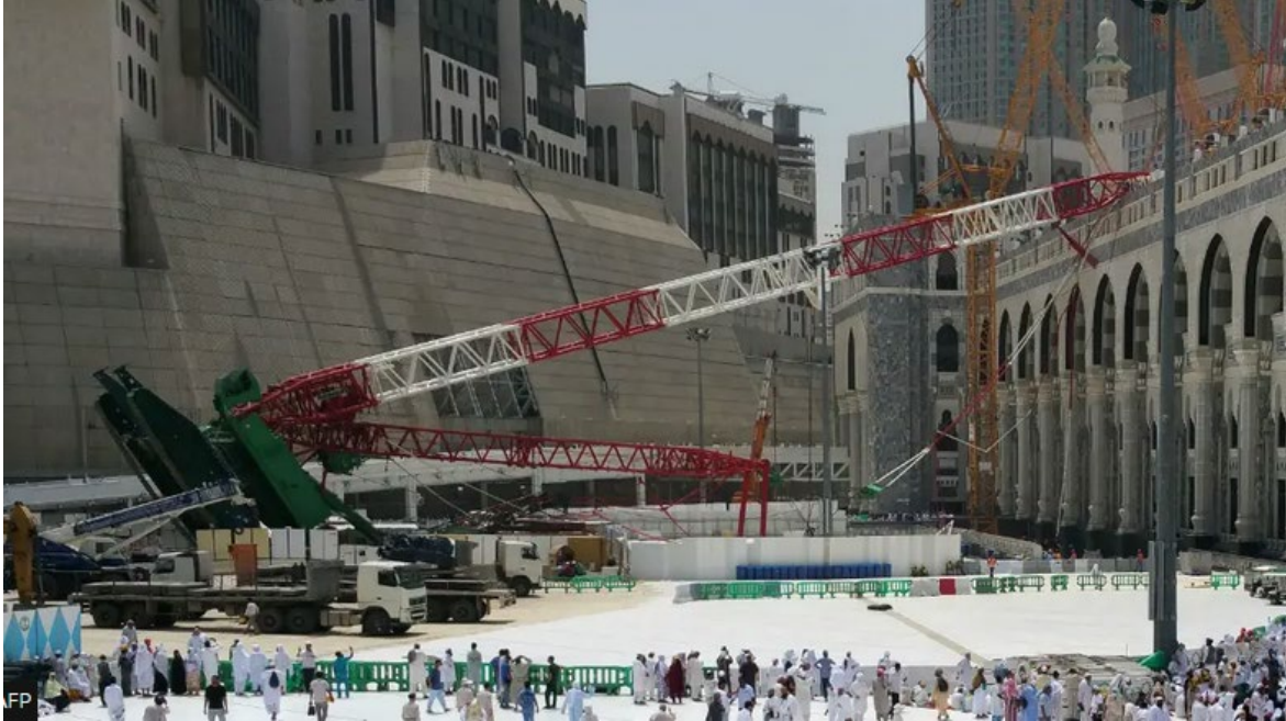
Figure 5-1. Fallen crawler crane at the Great Mosque in Saudi Arabia.
