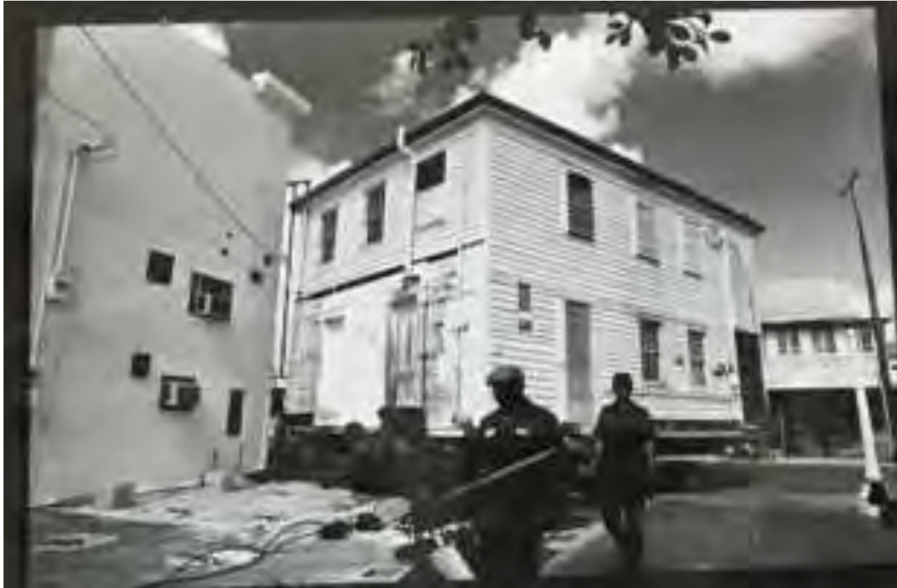
Rear of building to be located on the receiving site. Ed Swift III.
