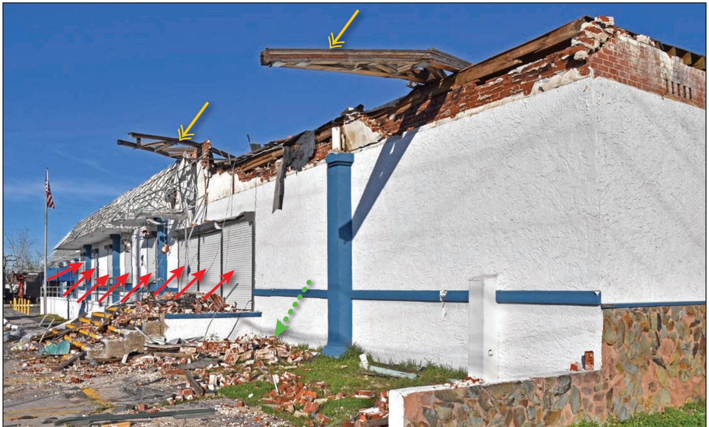
The red arrows indicate the retrofitted storm shutters. Two roof trusses are indicated by the yellow double arrows; the other trusses were blown off the roof. The green dashed arrow indicates collapsed brick.
