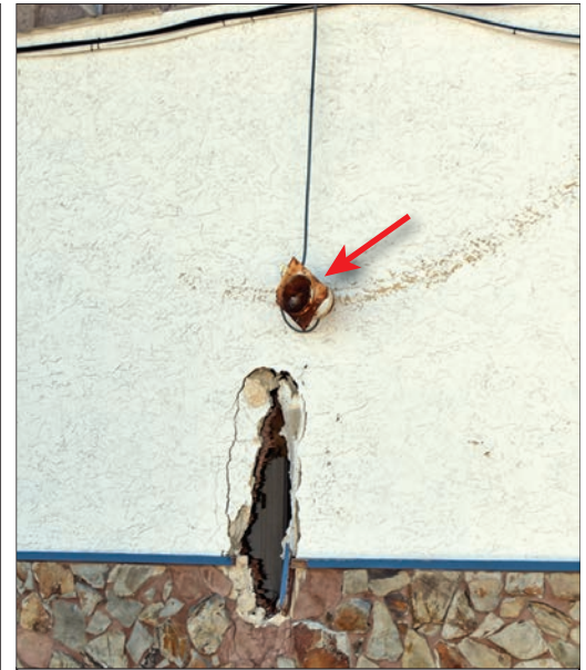
The white portion of the wall was stucco over metal lath over plywood over studs. The debris penetrated the interior gypsum board sheathing. The red arrow indicates a dangling light fixture that fell from the soffit.
