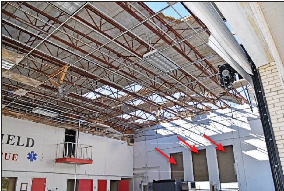
Figure 5: View of damaged roof after roof deck panels were blown off
