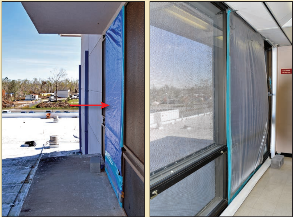
View of a window that failed under positive wind pressure
