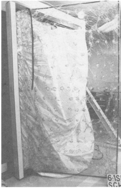
FIG. 9. Failure of Silicone Anchor Bead for Unconventionally Glazed System
