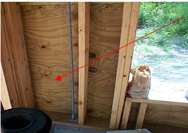
Photo C.3 shows: Threaded rod anchor system used in house. Anchors are placed in the foundation and the rods extend through the structure to the top plate to provide the “load path” to transfer uplift loads from the roof to the ground. Rods are placed on 4-foot centers (nominal) and are connected to roof framing where loads are high.
