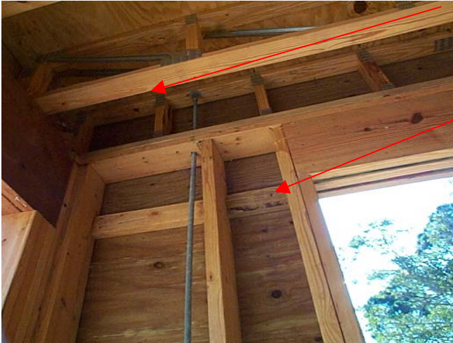
Photo C.4 shows: Additional picture of threaded rod connection passing through the top plate and floor above.
