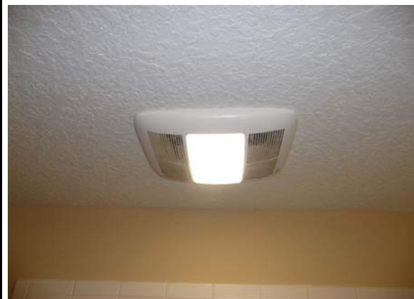
3-way switchable master bath exhaust fan with light (light comes on with fan; not separately controllable).
