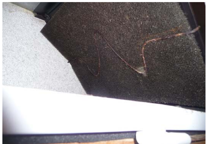
Energy recovery ventilator filter in fair condition.
