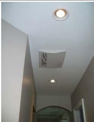
Ceiling mounted ERV in hall.
