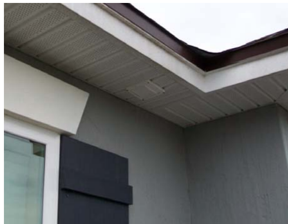
Outdoor air grille in second floor soffit.
