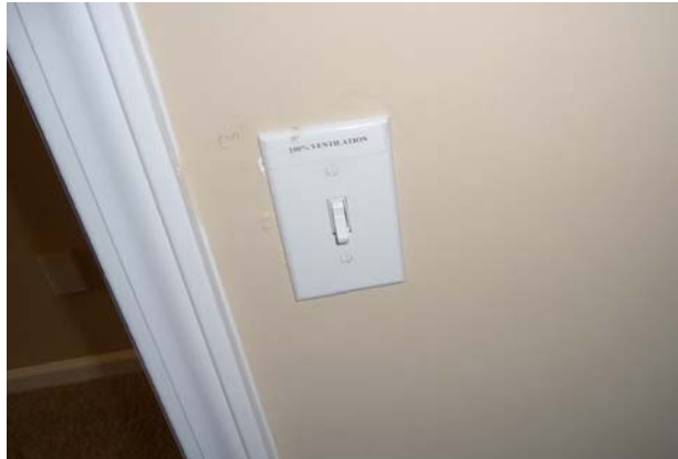
"100% Ventilation" switch in air handler closet likely used as part of 3-way switch to turn master bathroom exhaust fan on and off.
