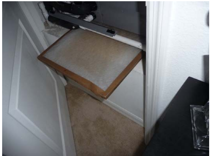
Filter at air handler for both AC and ventilation.
