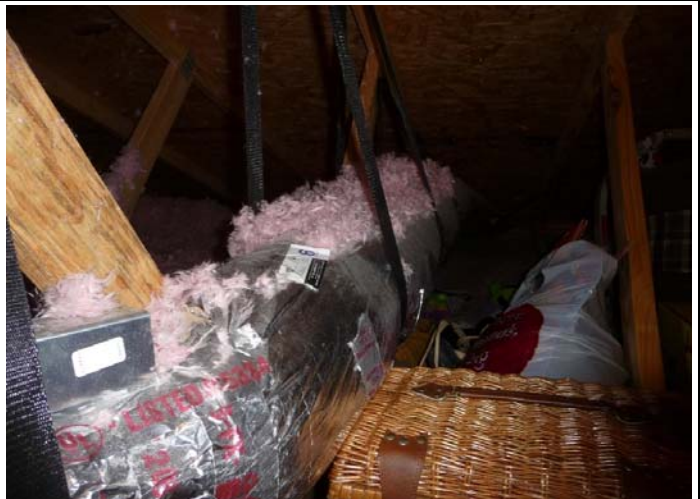
Outdoor air duct and damper in attic.
