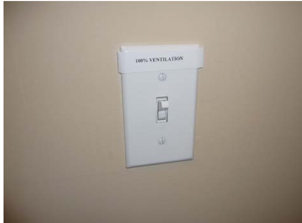
"100% Ventilation" switch likely used to turn on bathroom fan.
