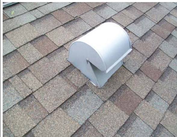
Outdoor air vent cap on roof.
