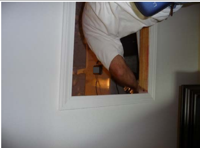
Ventilation controller located in attic; access via small bath.
