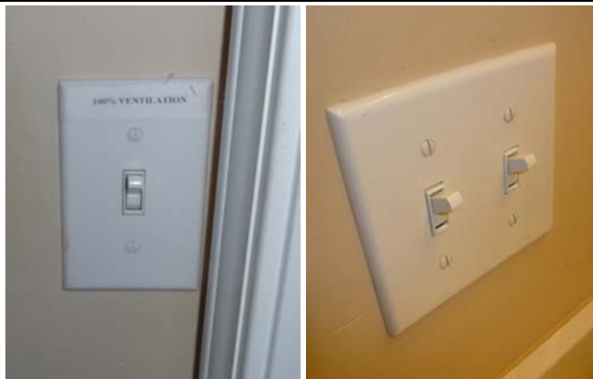
Either "100% Ventilation" switch in air handler closet (left) or master bath switch (right) can be used to turn bath fan on/off.
