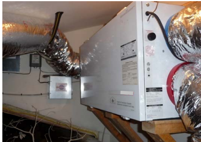
Energy recovery ventilator.
