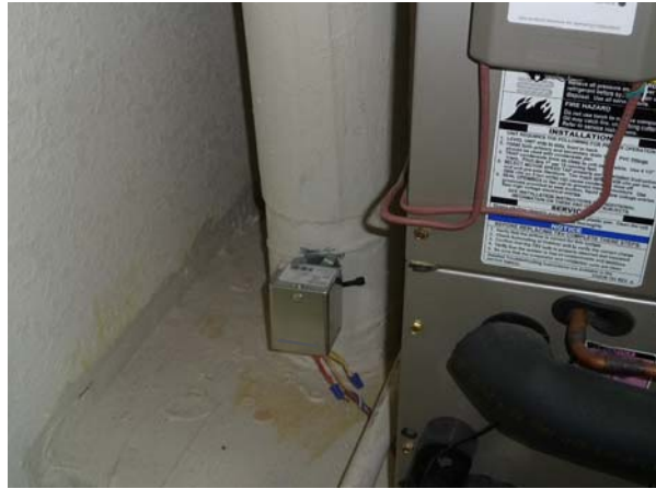
Outdoor air duct and damper controller next to air handler.
