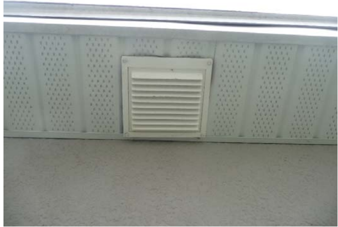
Soffit outdoor air intake grille.
