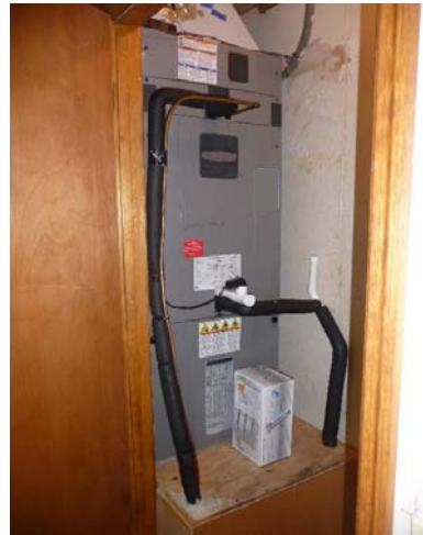
Air handler (ERV removed in 2014).
