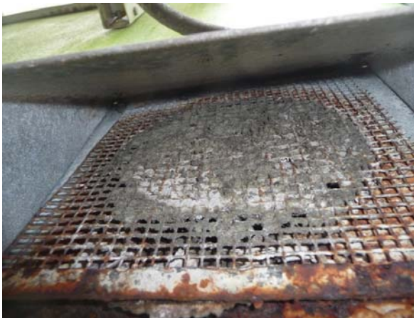
Dirty outdoor air intake.
