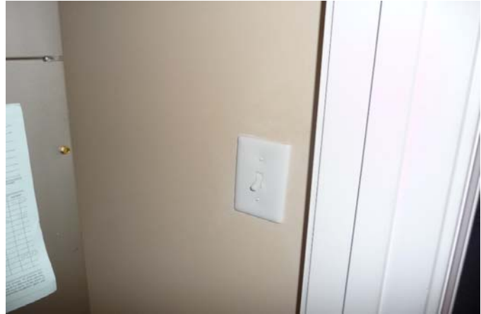
Switch in air handler closet likely used as part of 3-way switch to turn master bathroom exhaust fan on and off.
