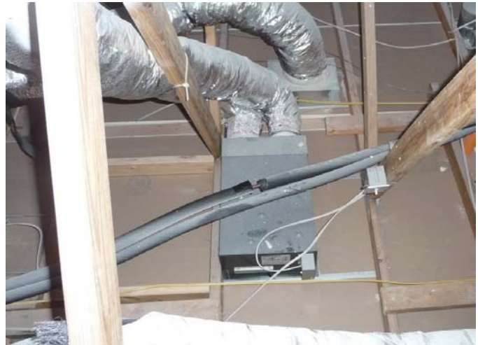
One of two ERV units with disconnect switch (right).
