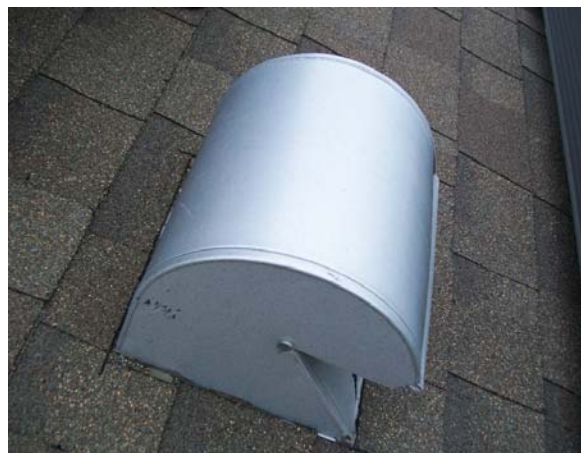
Outdoor air vent cap on roof.
