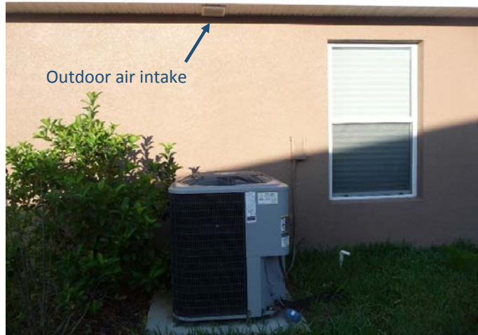
Outdoor air intake over AC condensing unit..
