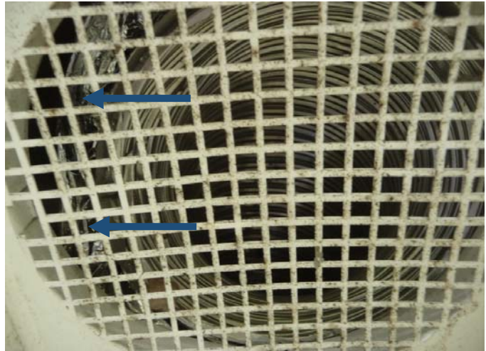
Outdoor air duct disconnected from grille.
