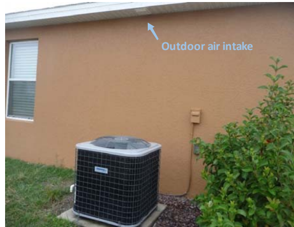
Outdoor air intake over AC condensing unit.
