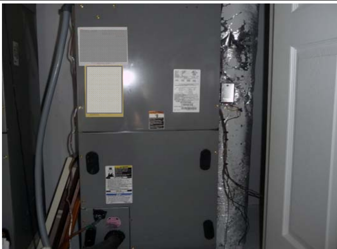
Air handler with outdoor air duct and damper.
