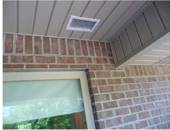
Outdoor air grille on front porch.
