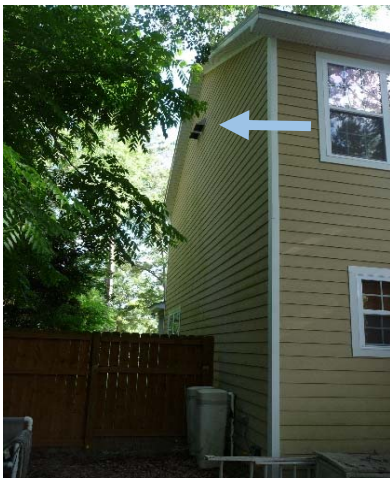
Supply and exhaust air grilles on 2nd floor wall.
