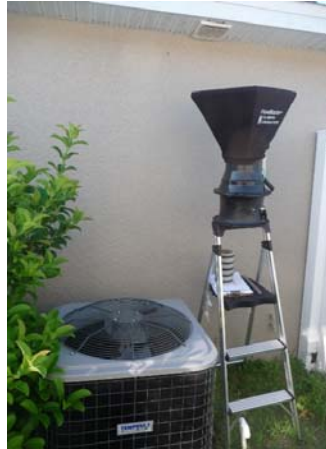
Outdoor air intake near condensing unit (also airflow tester).
