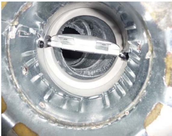
Open outdoor air damper visible from inside return plenum.
