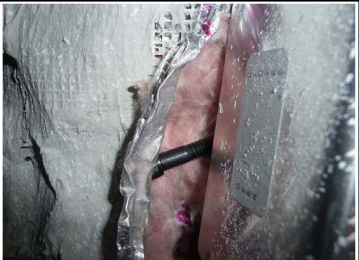
Closeup indicating outdoor air damper position.
