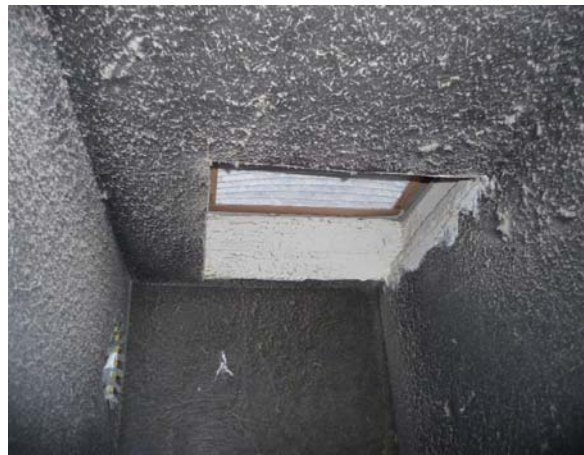
Outdoor air duct termination (left side) in return plenum.
