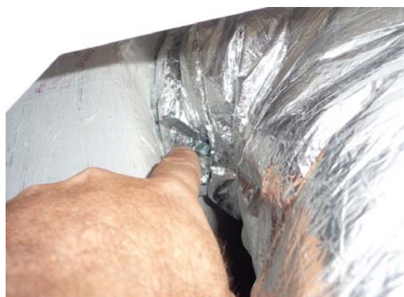
Manual damper for runtime vent system outdoor air duct found in closed position.
