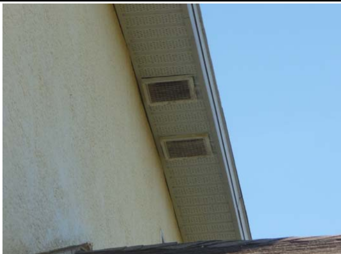
Outdoor air grilles in second floor soffit.
