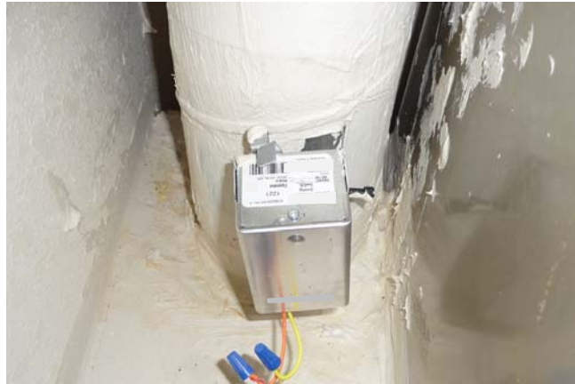
Outside air damper fixed open.
