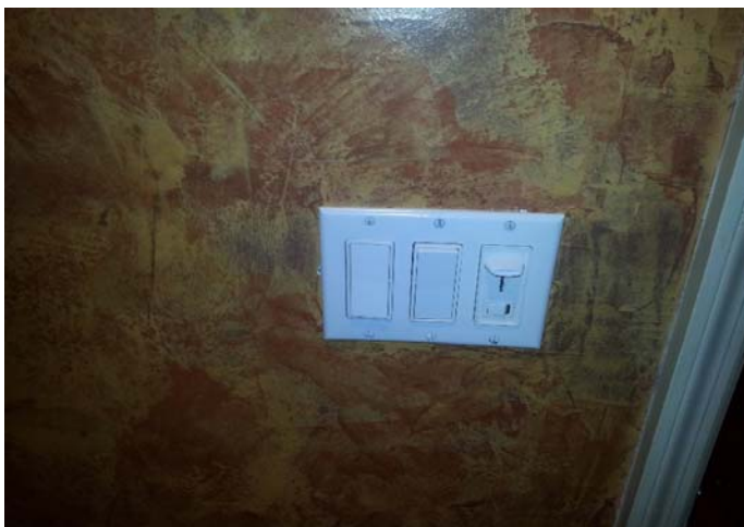
One of two bathrooms switches that turn the ERV on.
