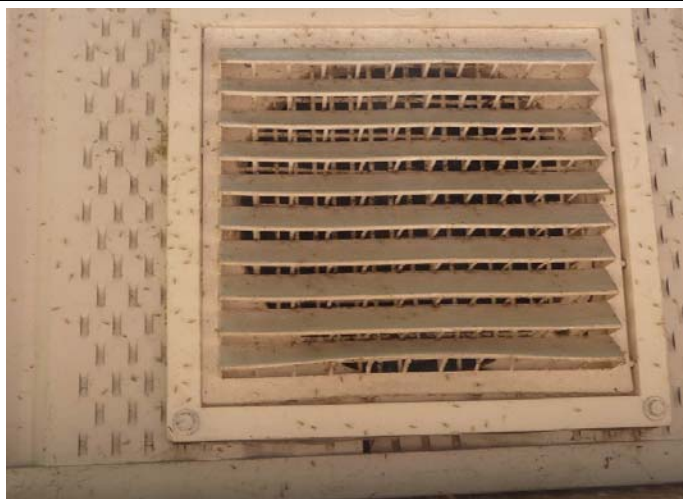
Relatively clean outdoor air grille.
