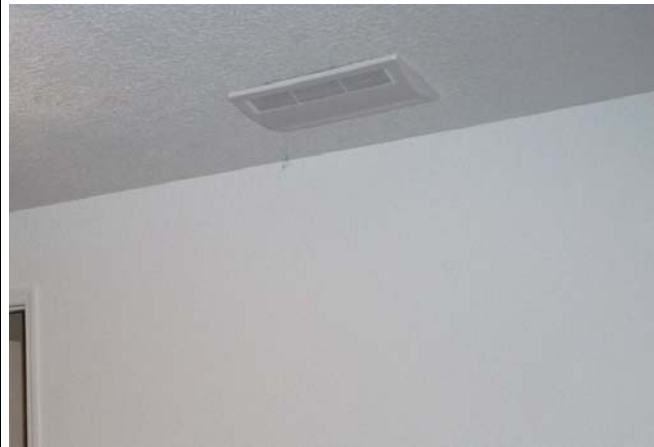
Energy recovery ventilator in living room.
