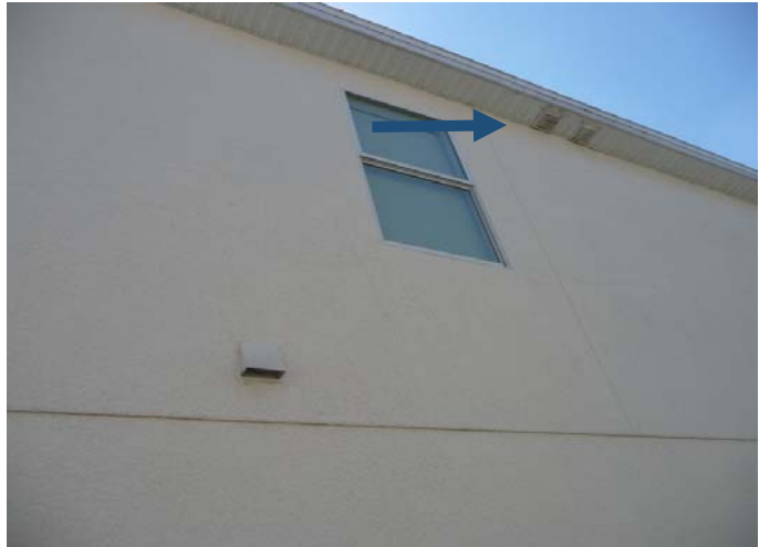
Outdoor air inlet grilles in second floor soffit.
