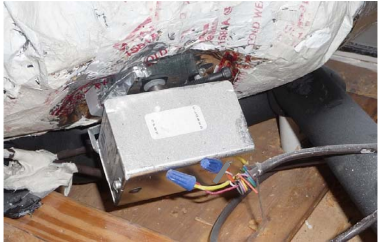
Outdoor damper in closed position.
