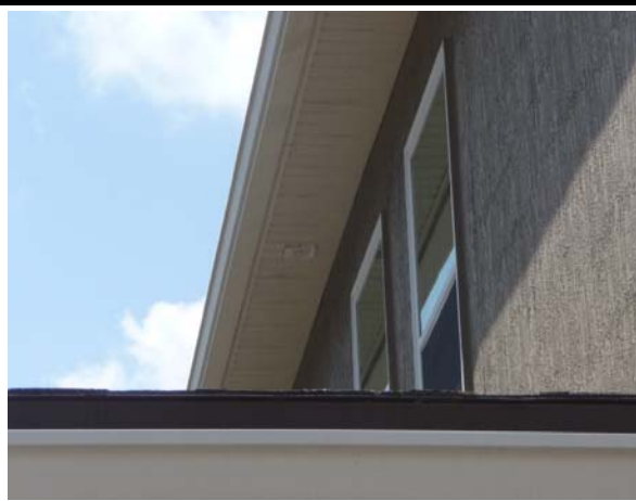
Runtime ventilation system outdoor air grille.
