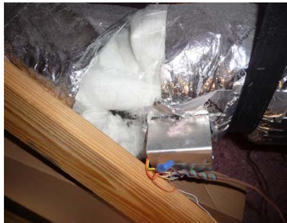
Ripped outdoor air duct outer jacket.
