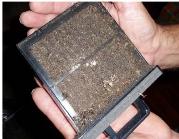
Dirty outdoor air filter.
