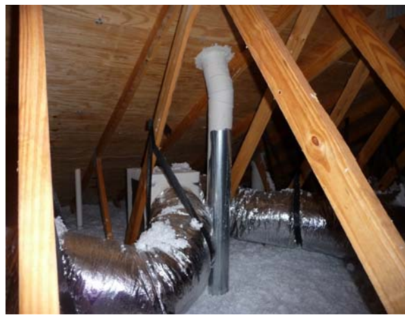
Outdoor air duct in attic is uninsulated.
