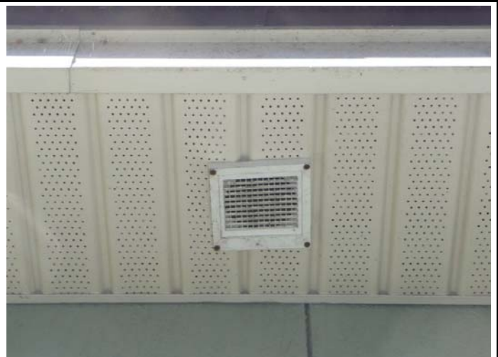
Runtime ventilation system outdoor air grille.
