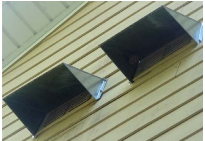
Close-up of supply and exhaust air grilles.
