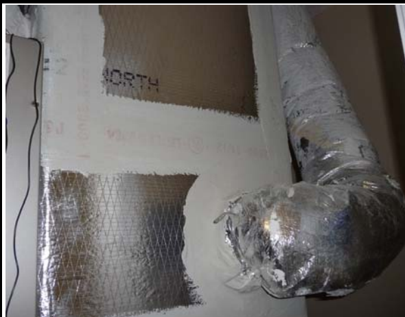
Runtime outdoor air duct with hard kinked turn at plenum.
