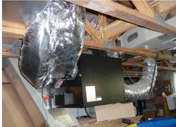
Energy recovery ventilator.
