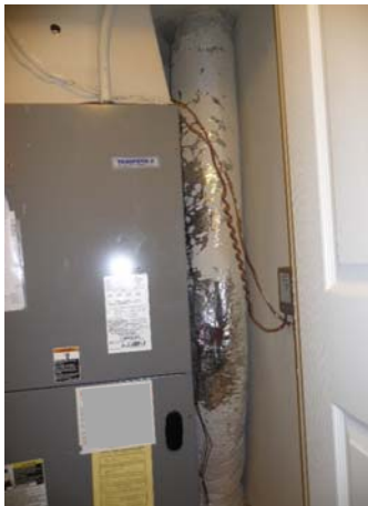
Air Handler and outdoor air duct to return plenum.
