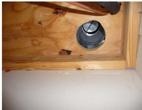
Outdoor air duct viewed from inside return plenum.
