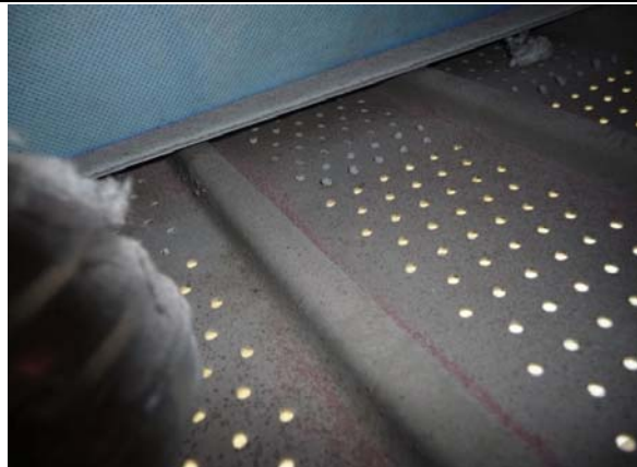
View from within exhaust discharge grille area due to disconnected duct (soffit should not be visible).
