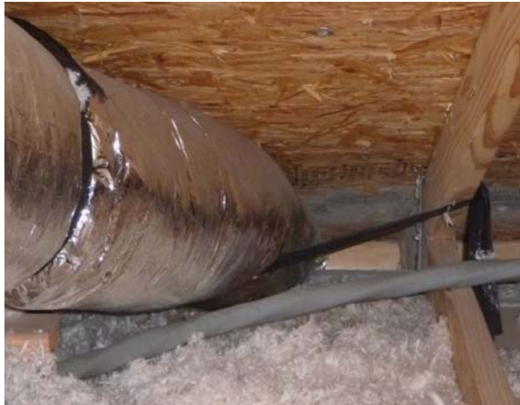
Partial outdoor air duct constriction at exterior wall.
