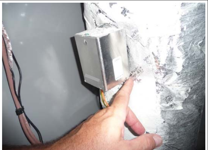
System 2 outdoor air damper inoperable.
