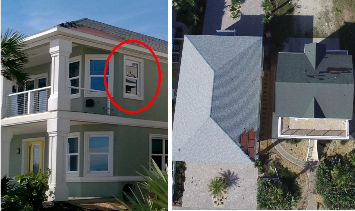
Figure 20: Ground view of broken window at 1424 S Ocean Shore Blvd (a) and aerial view of home with broken window and adjacent home which lost roof shingles (b).
