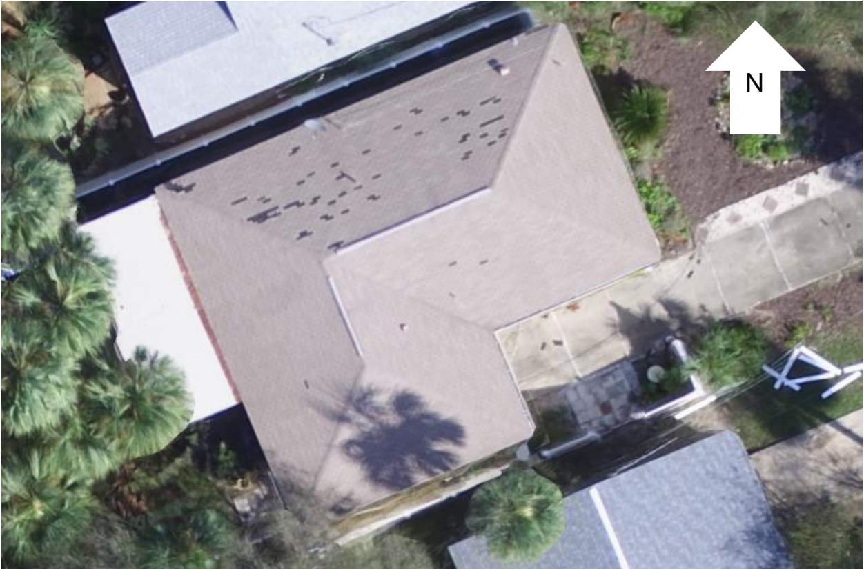
Figure 16: Scattered shingle damage to a one-story home at 1416 S Daytona Ave.
