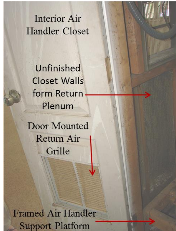
Figure 4. Interior air handler closet with no dedicated return air pathway. The unfinished closet walls (and poorly sealed ceiling) function as a return plenum.
