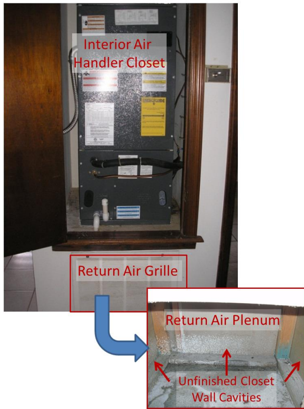
Figure 3. This air handler in an interior closet (left, top) is served by a return air plenum directly beneath (left, bottom) formed by the open, unfinished framing of the closet walls.
