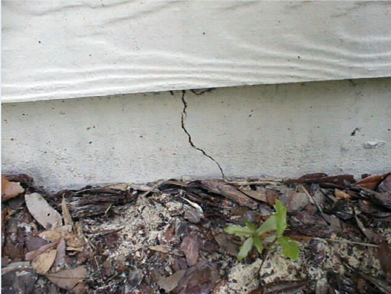
Cracks in foundation
