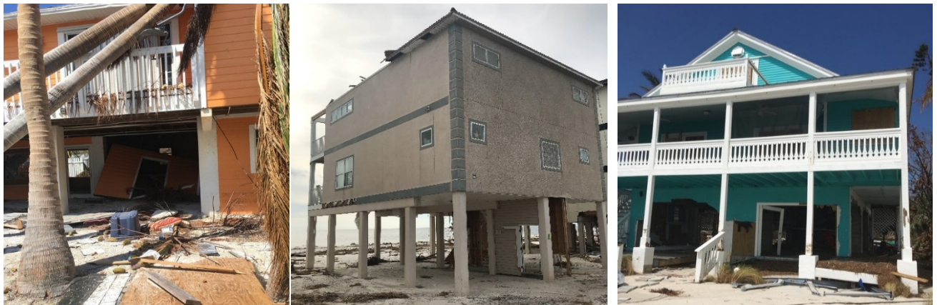
Figure 2. Ripping-off of the underside parts of the partially elevated houses recorded in Florida after the landfall of Hurricane Michael and Irma [8-9].
