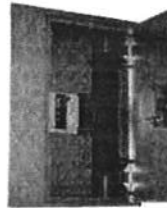
DISCONNECTS ARE PROVIDED
