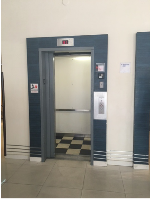
Elevator (open) from lobby
