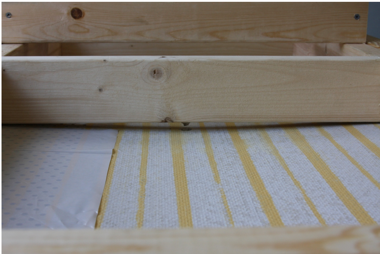
Figure 12. Observed Failure Modes
