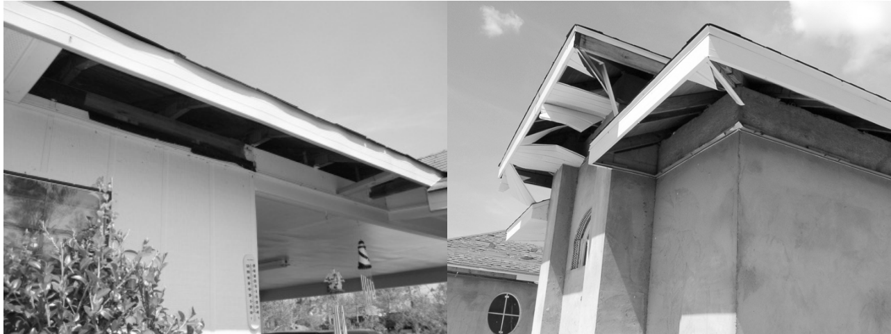
Figure 1. Soffit Damage Observed in Hurricanes Charley (2004) and Katrina (2005). Courtesy of Rick Dixon.
