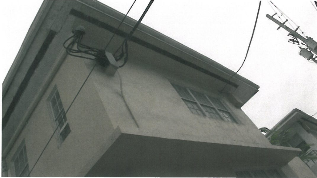
Northeast corner, electrical connection from transformer
