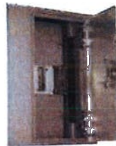
DISCONNECTS ARE PROVIDED
