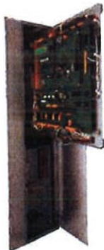
CONTROL PANEL IN DOOR JAMB
