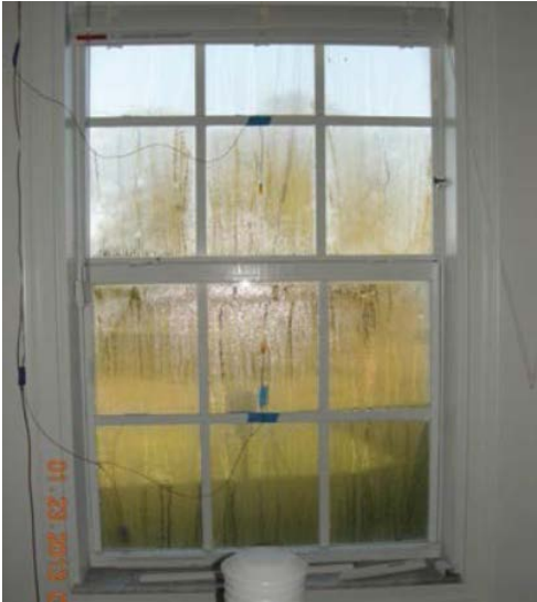
Figure 2 (figure from Vieira et al. 2013). Condensation on north-facing window in unventilated tight lab house January 23, 2013.
