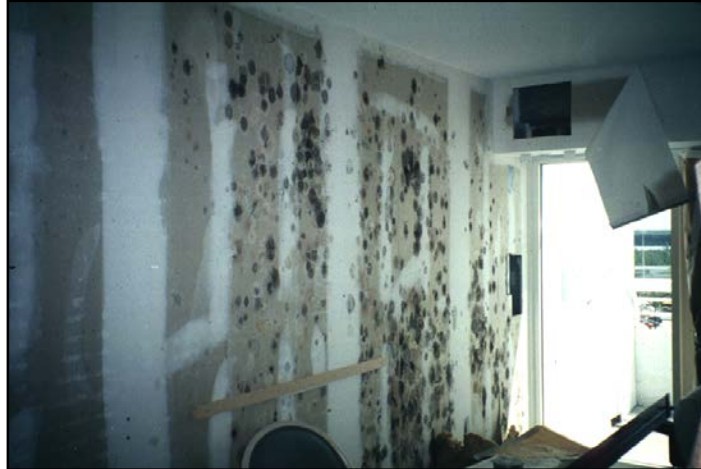
Figure 4. Mold covered wall resulting from a combination of factors including negative pressure and impermeable wall coverings.
