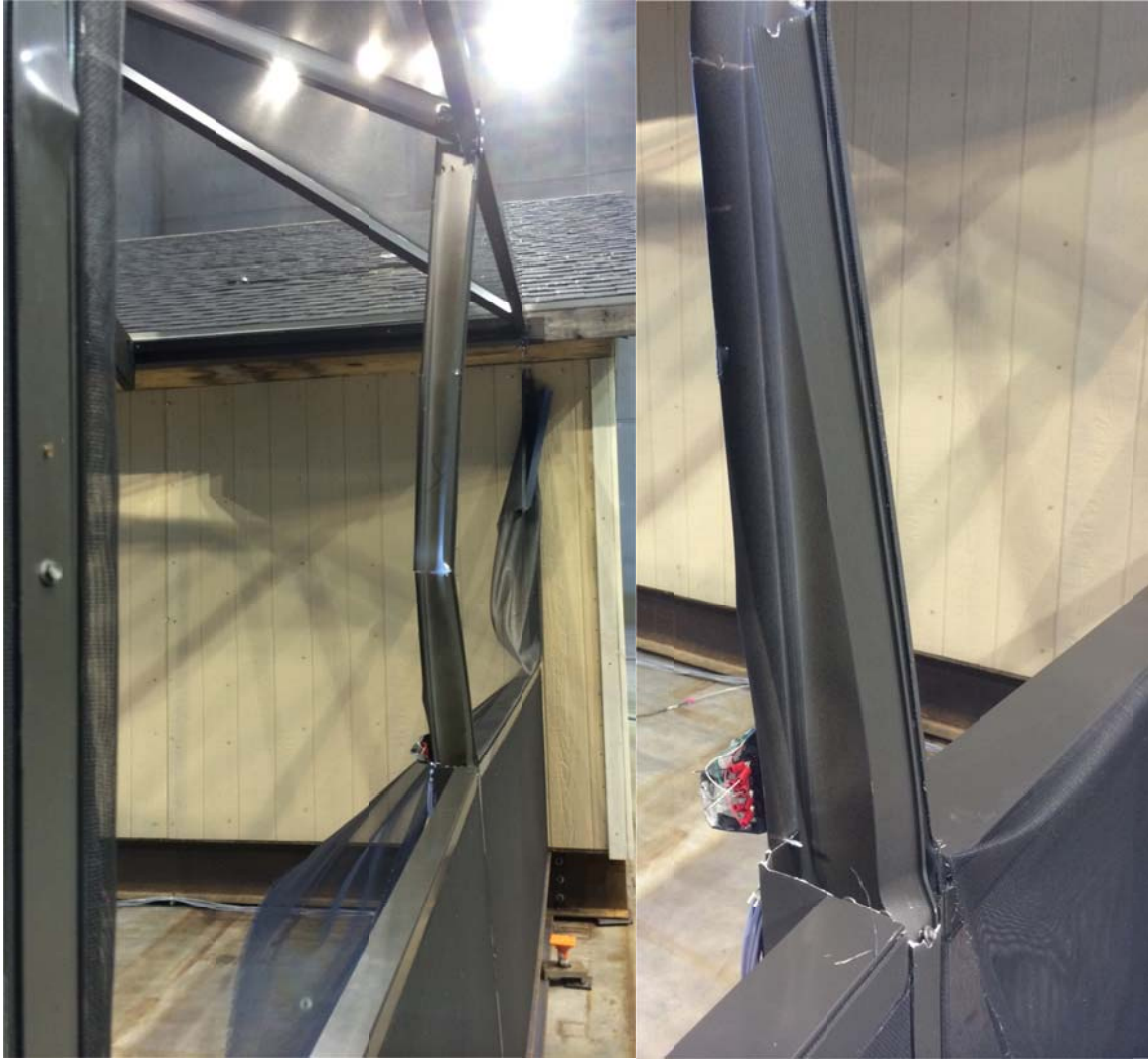
Figure 25. Failure of structural members after Run 31 (maximum wind speed = 100 mph)
