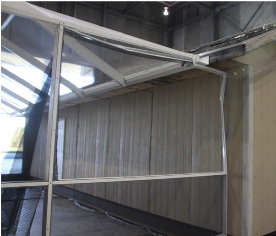
Figure 20. Failure of the structural members after Run 30
