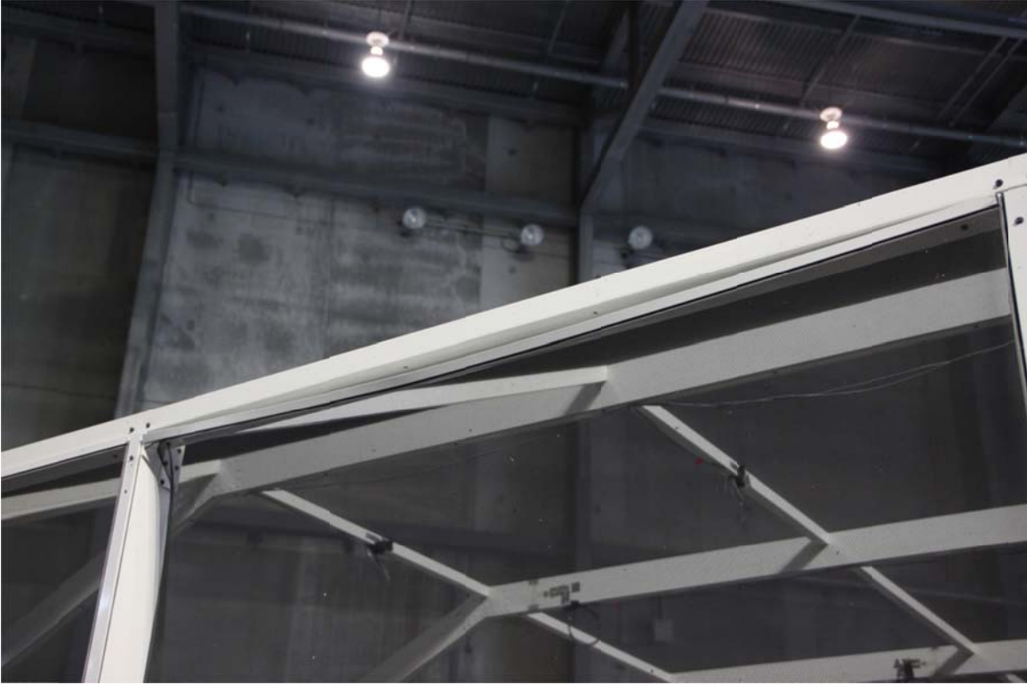
Figure 17. Partial failure of the screen attachment due to the pullout of screws (after Run 27)
