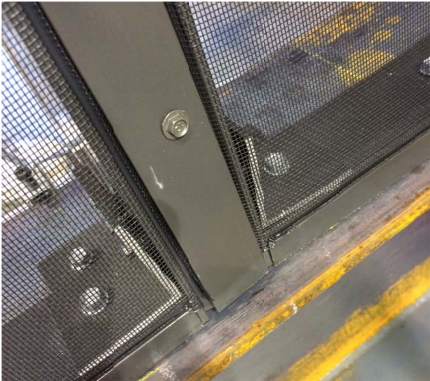
Figure 27. Local failure of brackets at the base of the post (windward wall for 0 degree wind angle, third post from the left)
