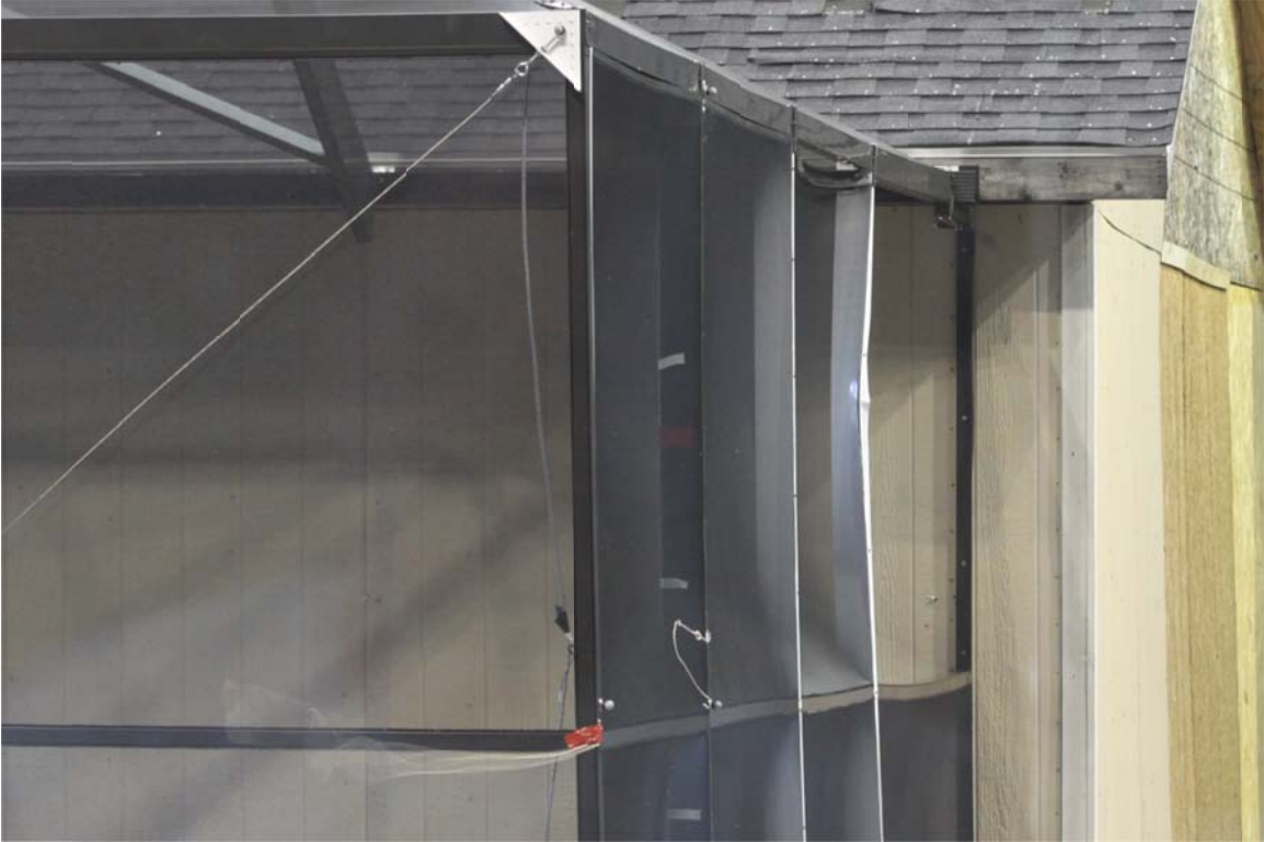
Figure 26. Reproduction of failure of the column in Run 37: unbalanced loading with the failed screen attachment led to the failure of the column
