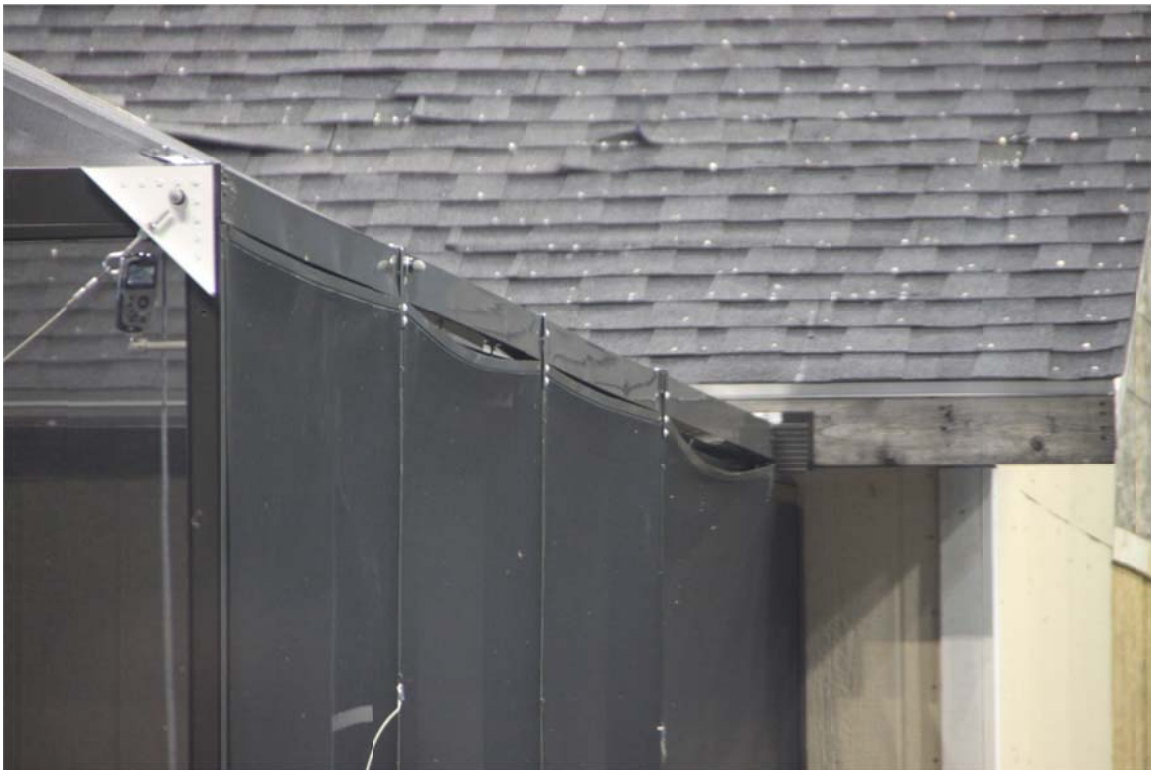
Figure 22. Partial failure of the screen attachment during Run 27 (maximum wind speed = 80 mph)
