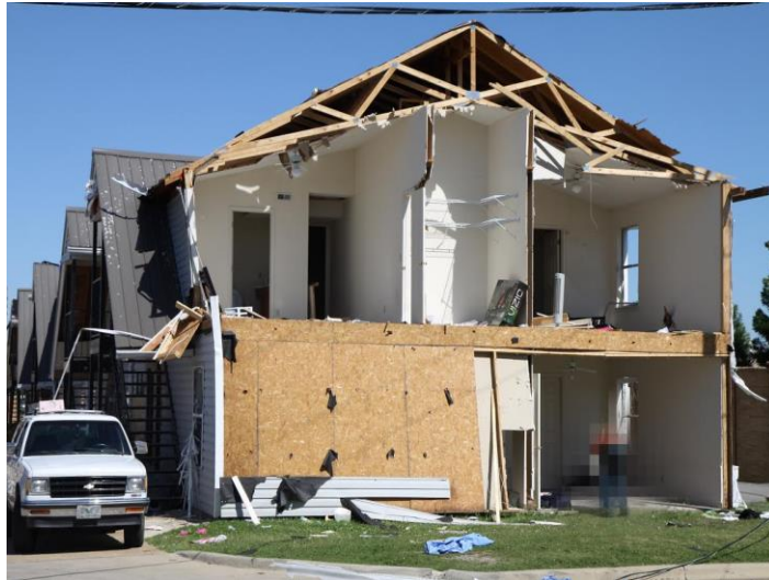
Figure 21: Wall connection failures from tornado damage
