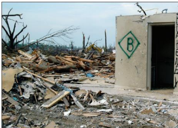
Figure 16: A hardened room in a residence Tuscaloosa, AL whose door failed in the April 27, 2011 tornado (source: FEMA (2012))
