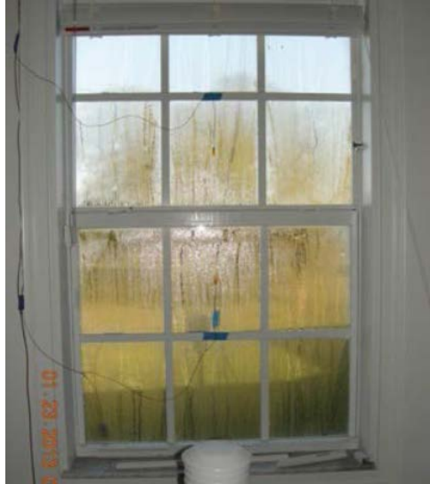
Figure 2 (figure from Vieira et al. 2013). Condensation on north-facing window in unventilated tight lab house January 23, 2013.
