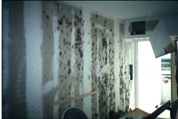
Figure 4. Mold covered wall resulting from a combination of factors including negative pressure and impermeable wall coverings.
