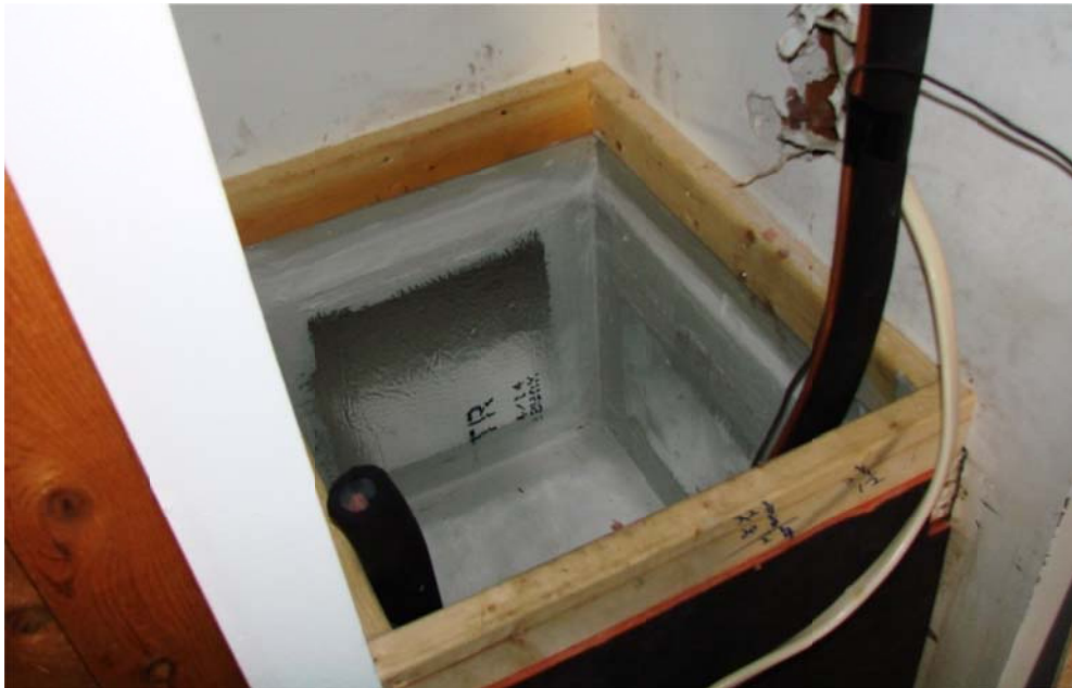
Figure 14 New duct board lining provides an air barrier to separate the return air stream from adjacent open wall cavities.
