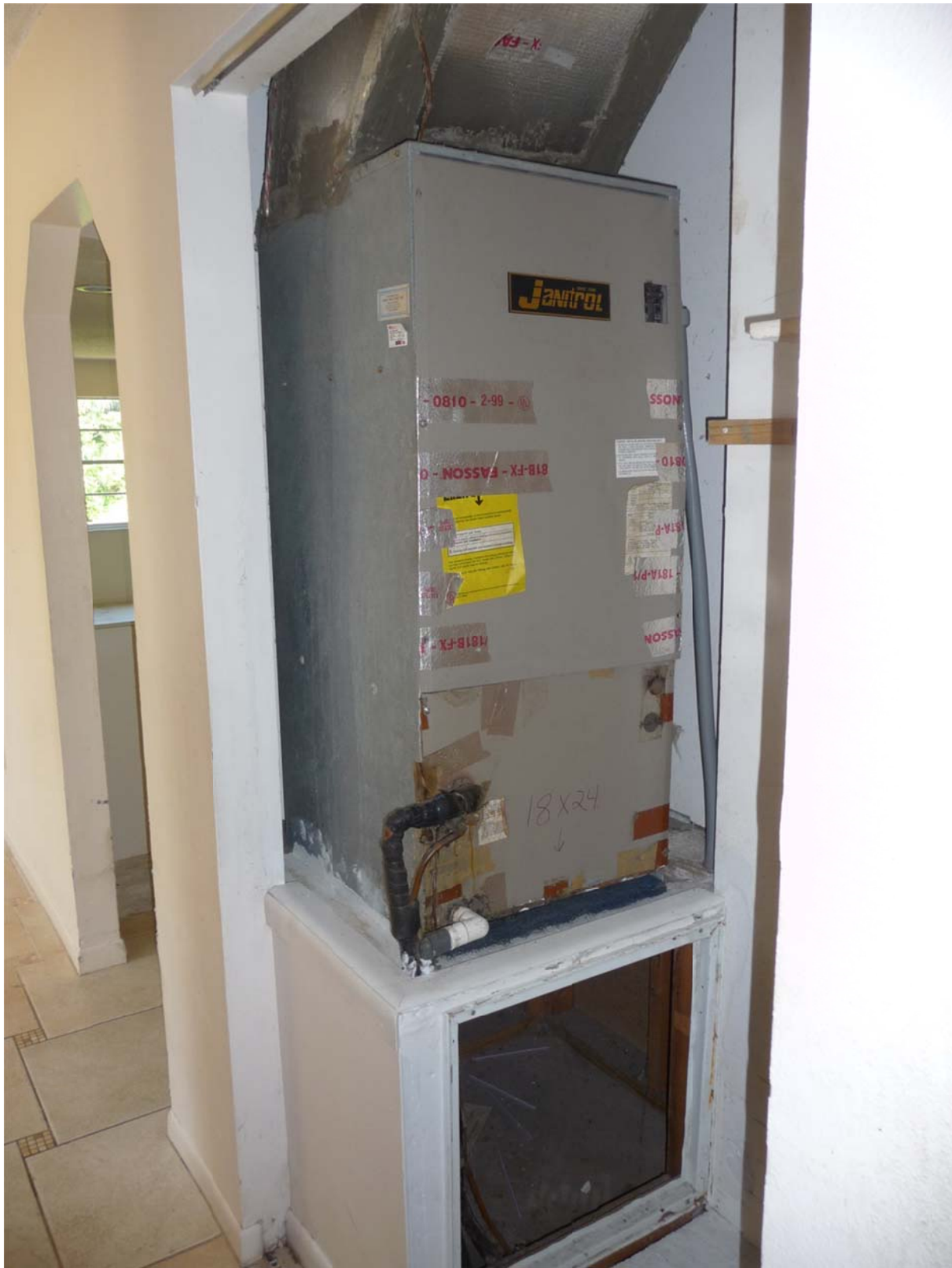
Figure 18. Note the open wall cavities in the return plenum and the raised plywood floor in the closet (in the lower right corner of the image)
