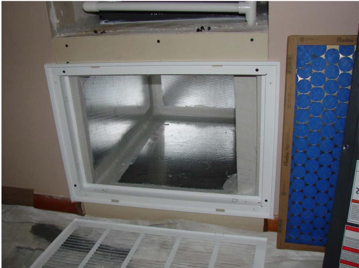
Figure 28. Repaired platform return plenum with duct board air barrier sealed at edges.
