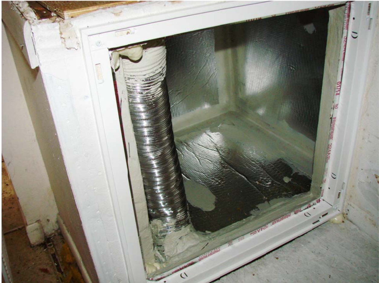
Figure 22. Repaired return plenum lined with duct board air barrier sealed with mastic at all edges.
