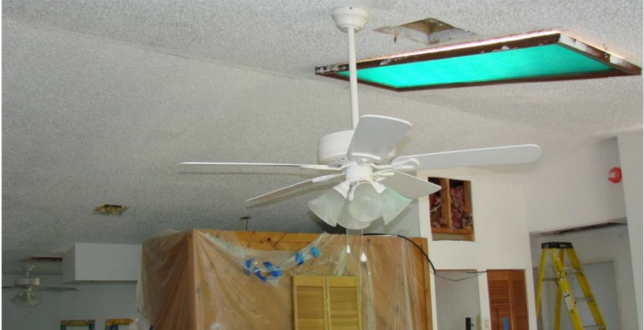
Figure 13. The hole in the wall over the air handler closet was cut to facilitate supply plenum installation. Also note the living room supply, to be relocated during repair.
