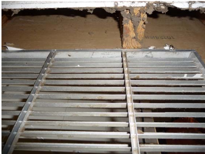
Figure 6. Looking up into the wall cavity from the wall-mounted return air grille. This wall cavity is part of the return air plenum because there is no air barrier separating it from the return air flow path.
