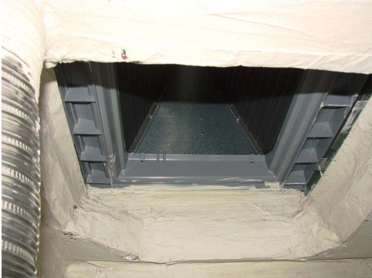
Figure 123. Return air entry to air handler seen from inside the return plenum. Joint between plenum, platform, and air handler is thoroughly sealed with mastic.
