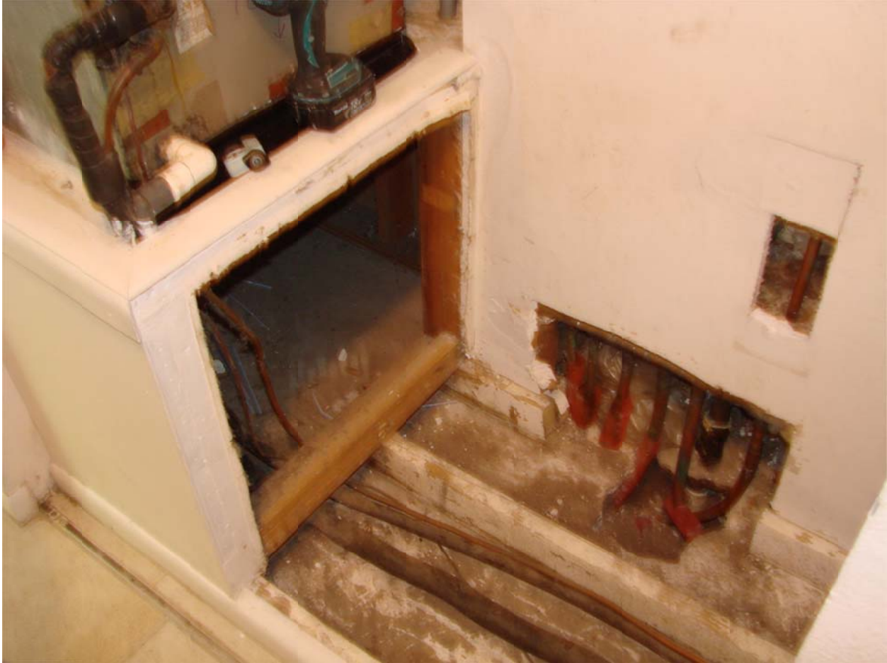
Figure 19. Raised closet floor created a plumbing chase for refrigerant line, condensate drain line and other plumbing run. Chase is fully connected to return air plenum at pipe penetrations.
