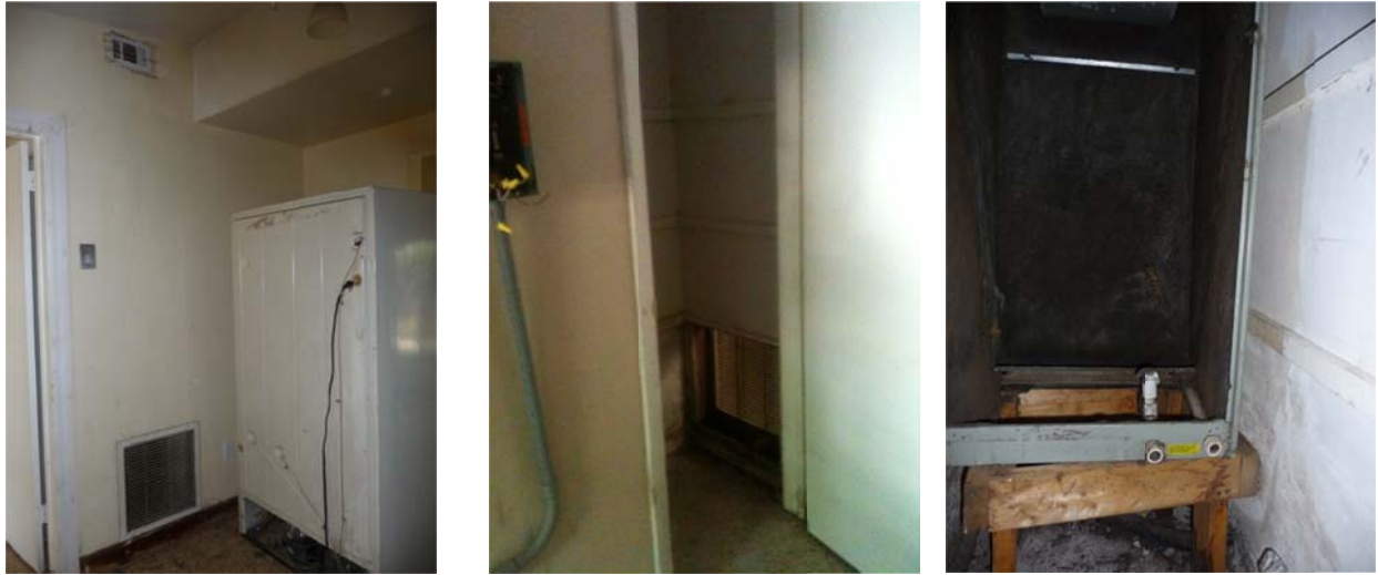
Figure 5. The entire air handler closet serves as the return plenum. Left: Central (only) return air grille mounted in wall between kitchen and air handler closet. Center: Air handler closet showing back of return air grille. Right: Inside the air handler closet, to the left of the door, showing air handler mounted on free-standing wooden supports.
