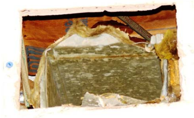
Figure 7. Disconnected supply duct
