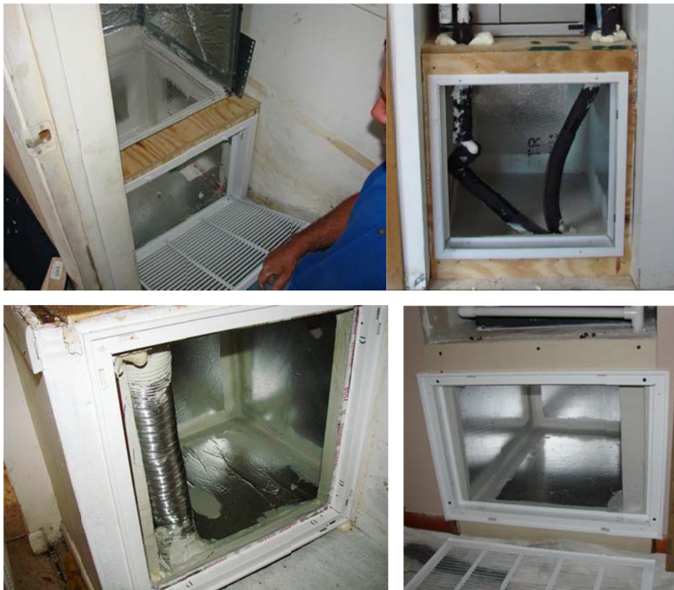
Figure 33. Air barrier lined return plenums in Test Houses (left to right) 1962, 194, 261, and 223.
