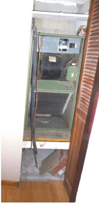
Figure 26. Air handler closet with open frame platform return plenum.
