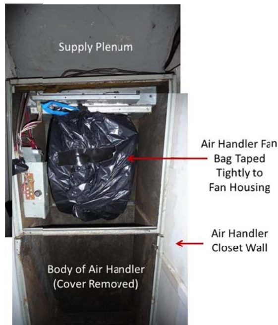
Figure 8. Return portion of air distribution system isolated from the supply by sealing around the air handler fan with a plastic bag taped at all edges.
