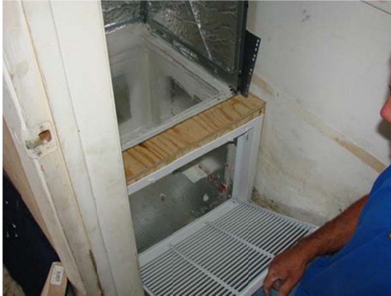
Figure 9. Filter-back return grille installed on new platform return in existing air handler closet.
