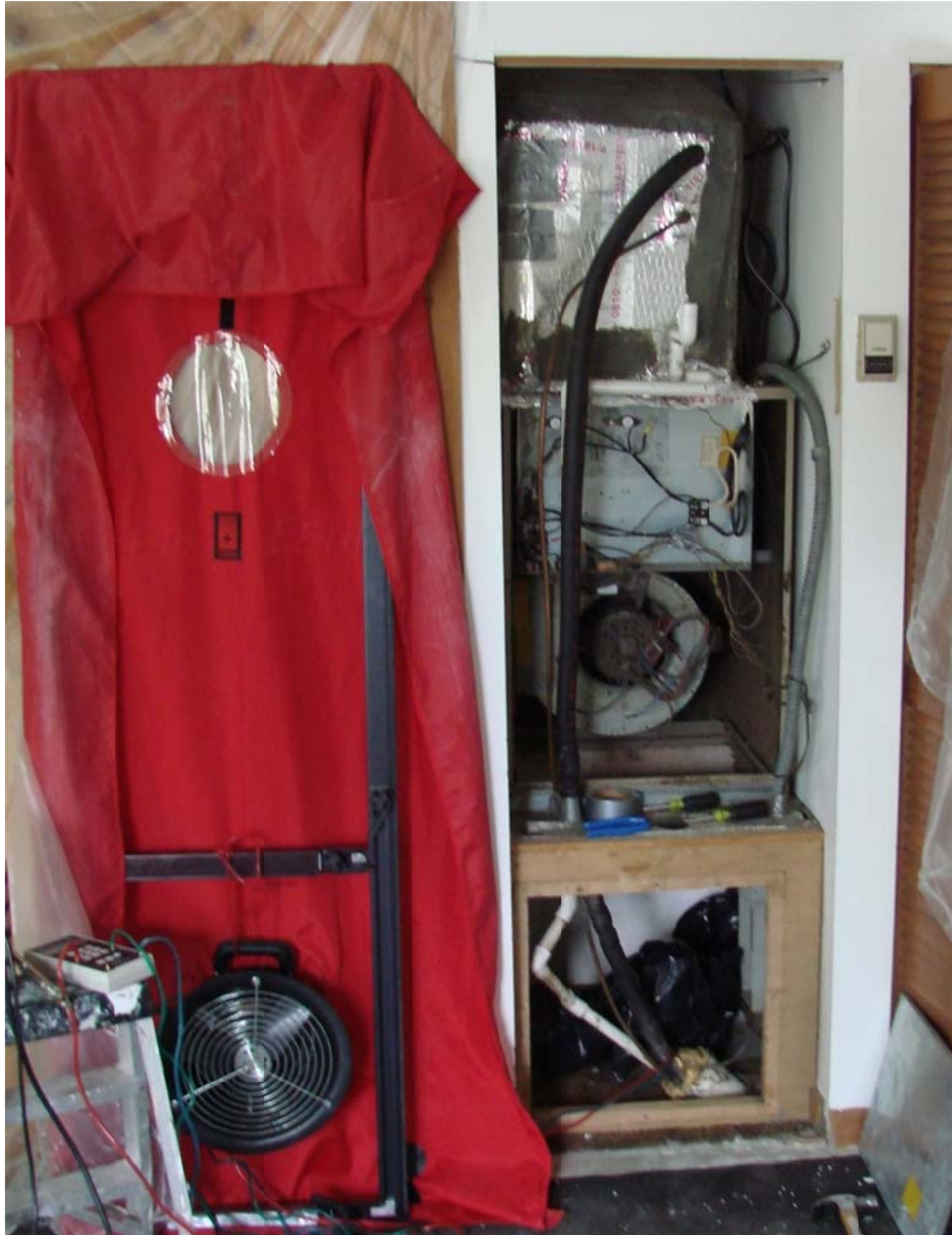
Figure 12. Air handler mounted on an open frame platform
