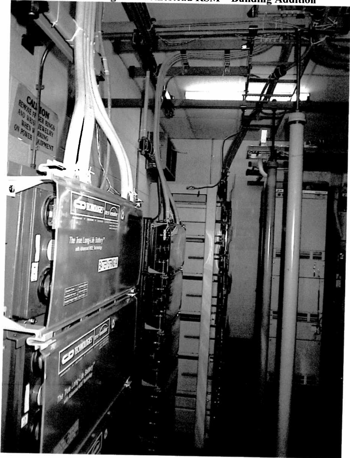
TELEPHONE EQUIPMENT AREA
