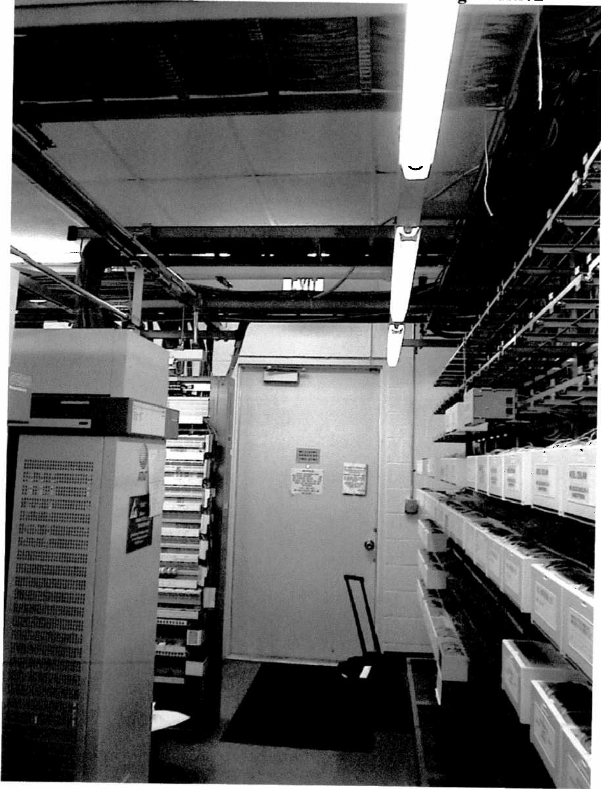
TELEPHONE EQUIPMENT AREA
