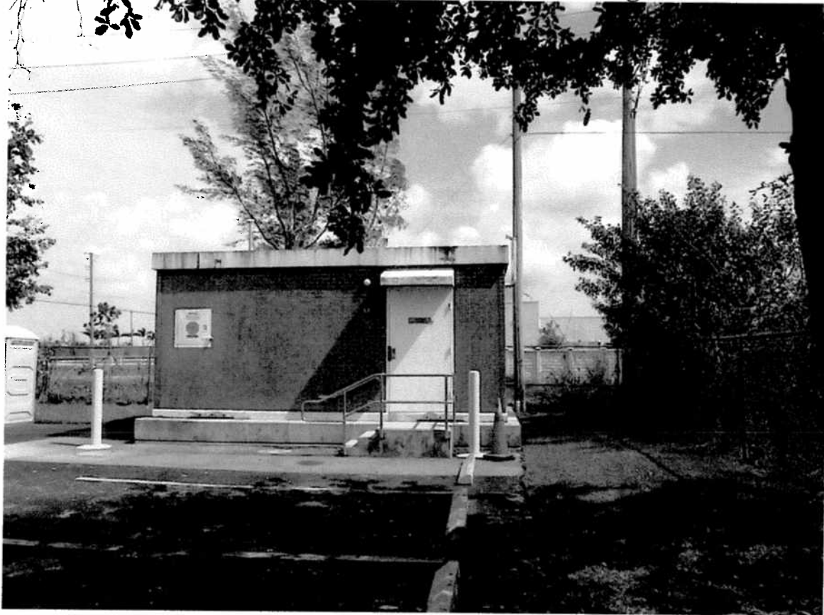
VIEW OF GENERATOR FACING EAST
