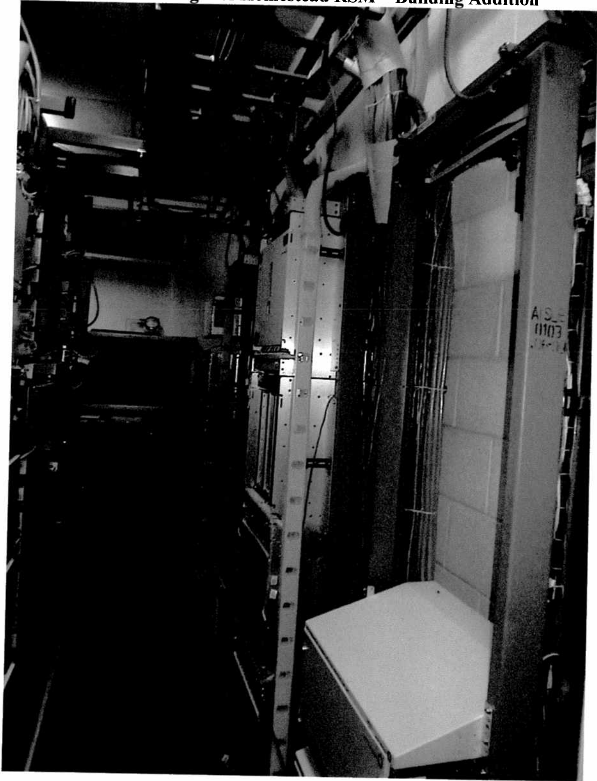
TELEPHONE EQUIPMENT AREA
