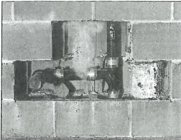
Figure P2503.5.2(2) SMOKE INDICATING PRESENCE OF LEAK (Photo courtesy of Hurco Technologies, Inc.)
