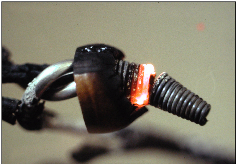
FIGURE 1 - ALUMINUM WIRE SPLICES MADE WITH TWIST-ON CONNECTORS CAN BE DANGEROUS. The use of most types of twist-on connectors with aluminum wire can lead to hazardous results. This twist-on pigtail connection (two #10 aluminum wires with one #12 copper wire, in a 20-amp circuit), made with a twist-on connector that was UL listed for use with aluminum wire at the time, remains electrically functional in the circuit, but it becomes extremely hot whenever a significant amount of current flows. The heat has deteriorated the insulation on both the connector and the wires. In this photo, a portion of the connector's spring is red hot, at current well below the circuit rating.
