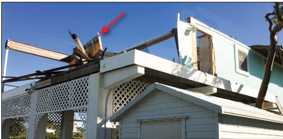
The screened porch and portion of the exterior wall, which is painted orange and indicated with the red arrow, remained standing. There is a missing wall section between it and the west-facing exterior wall. Same house as Figure 4-3.
