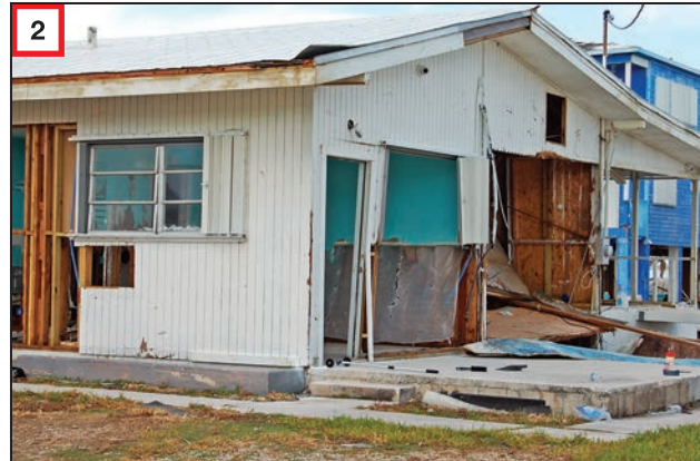
Inundation, water velocity, and debris damage to buildings situated farther from the shoreline.
