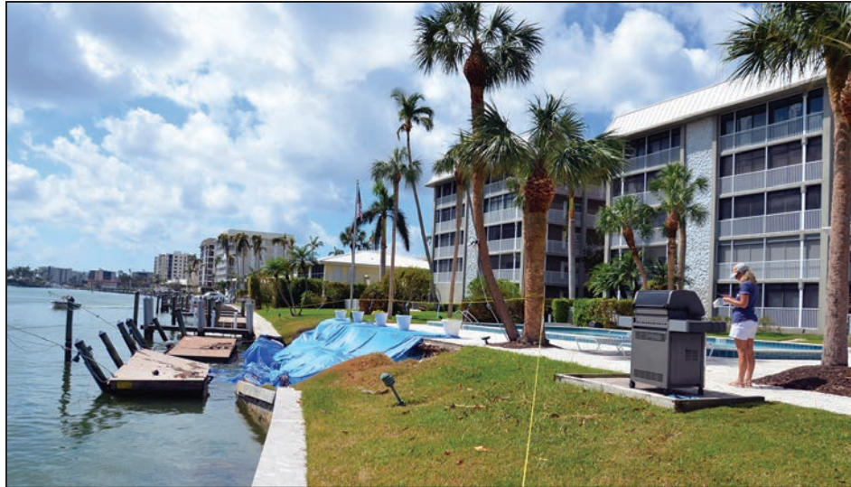
Figure 3-27: Failure of bulkhead (anchor system) (Naples, FL)
