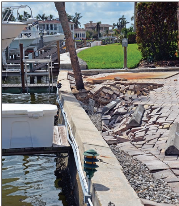
Figure 3-28: Bulkhead toe failure (insufficient embedment) (Naples, FL)
