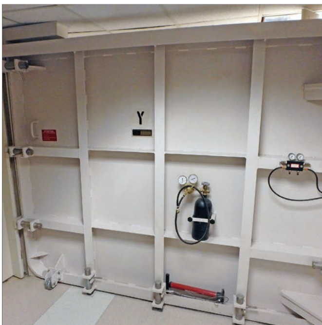
Figure 7: Flood gate with an air tank and a hand pump as a redundancy measure to inflate gaskets
