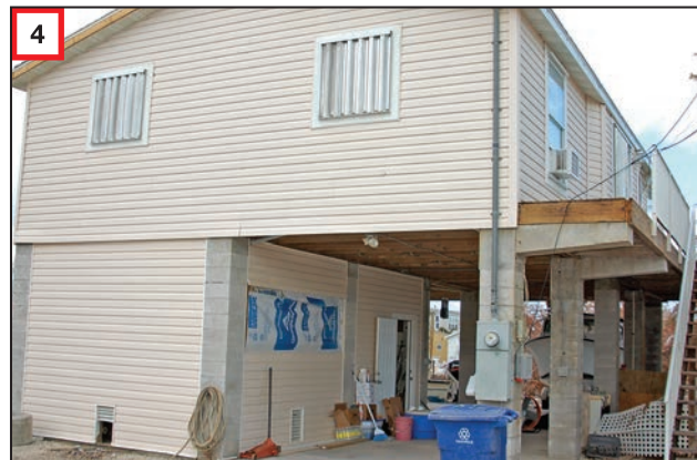
Minor enclosure damage to newer, elevated house situated away from the shoreline.
