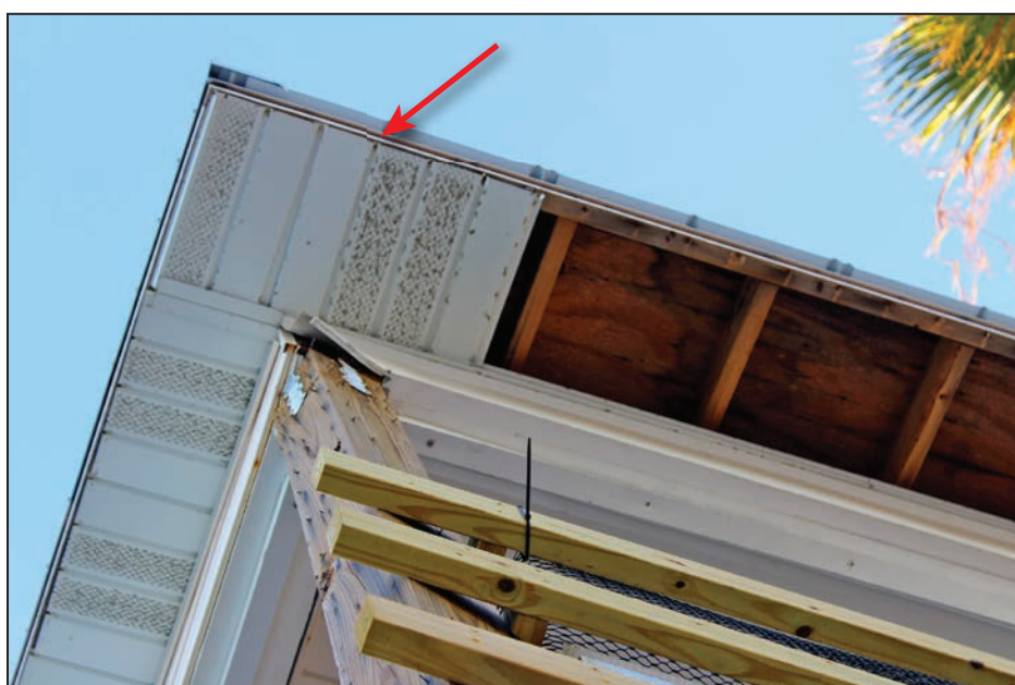
The red arrow shows direct attachment of soffit to framing along the outside edge of eaves only; panels are secured by a channel only above the porch opening.
