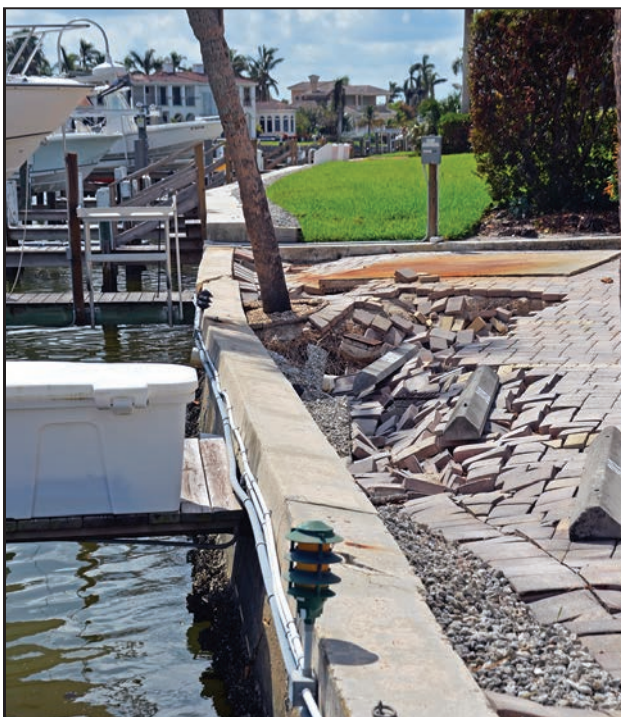
Figure 3-28: Bulkhead toe failure (insufficient embedment) (Naples, FL)
