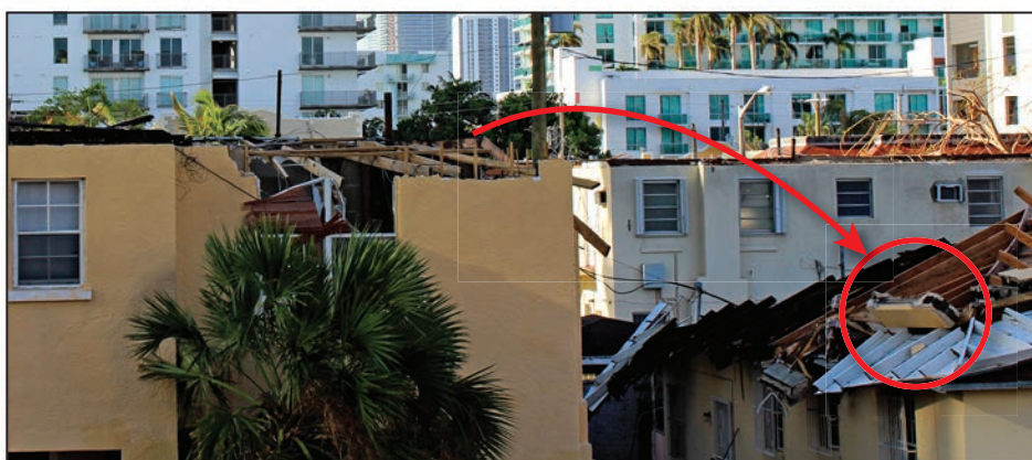
Figure 4-2: Residence where a roof-to- wall connection failed (EWS = 78 mph; EDWS = 169 mph) (Miami)
