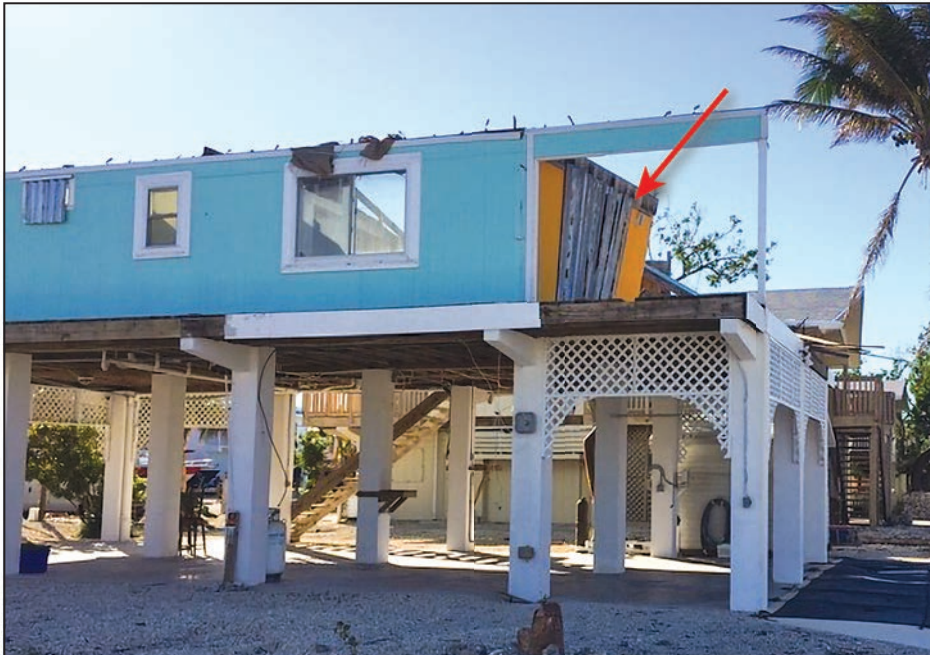
One section of the north-facing exterior wall (painted orange, indicated with the red arrow) adjacent to screened porch remained in place. Same house as Figure 4-3.
