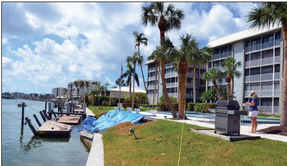
Figure 3-27: Failure of bulkhead (anchor system) (Naples, FL)
