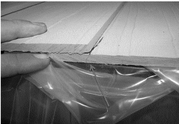
Typical fracture noted at siding ends
