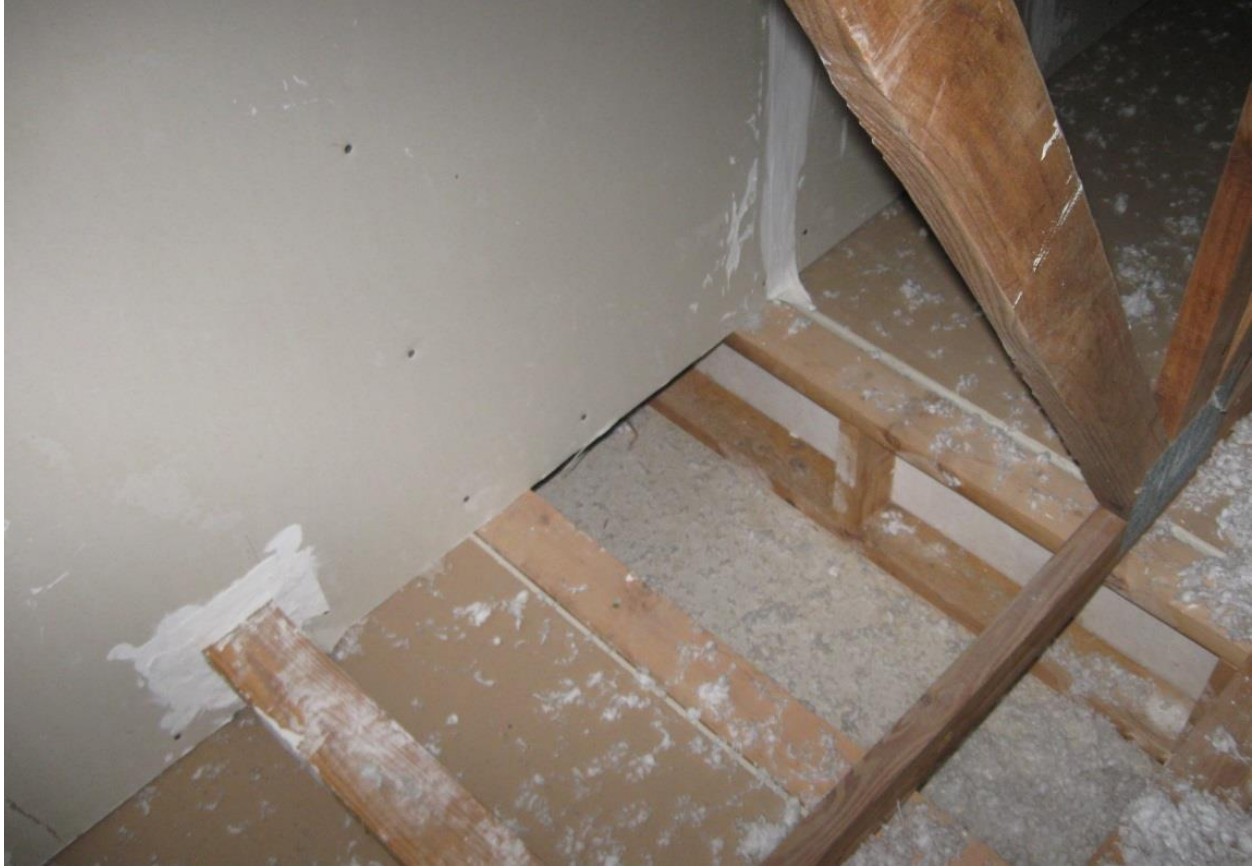
Picture 11 – Building 12 Deficiency.
