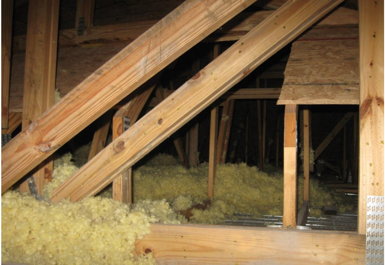
Picture 08 – Building 6 Deficiency.
