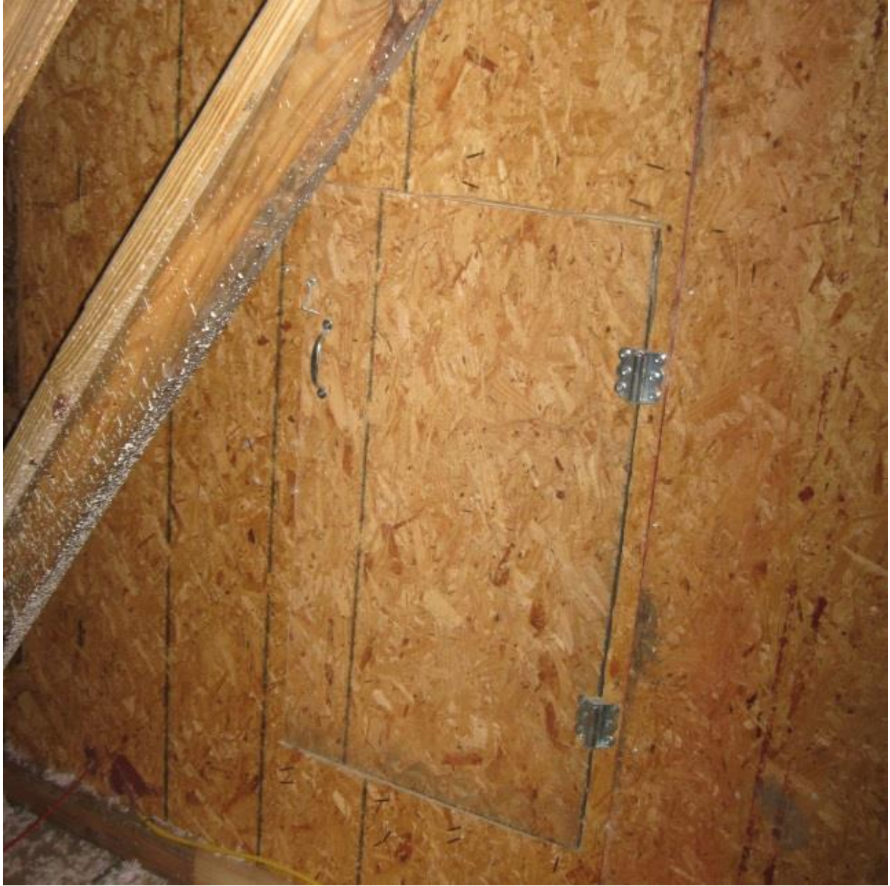
Picture 02 – Typical Door in Plywood Draftstopping
