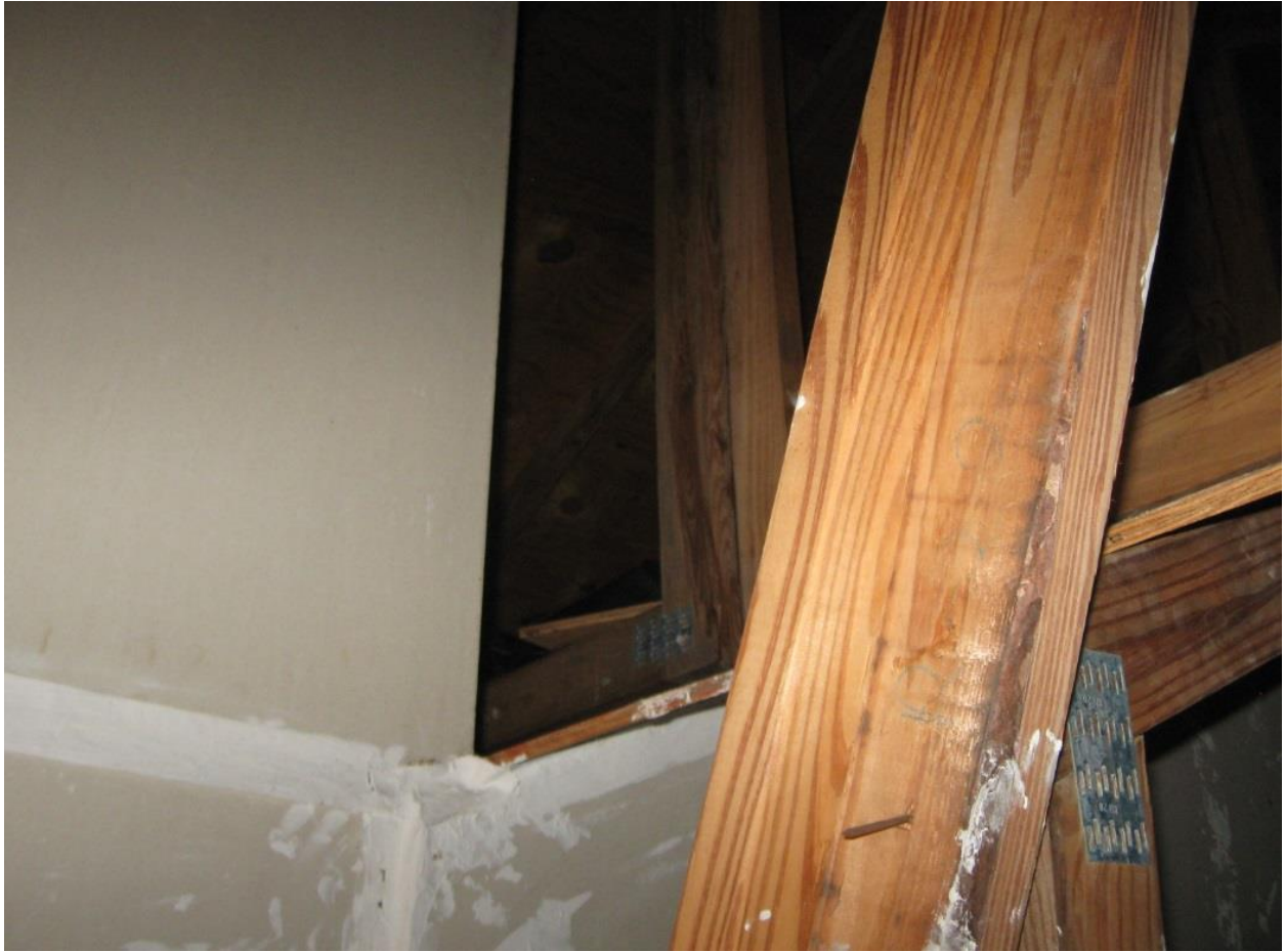
Picture 10 – Building 12 Deficiency.
