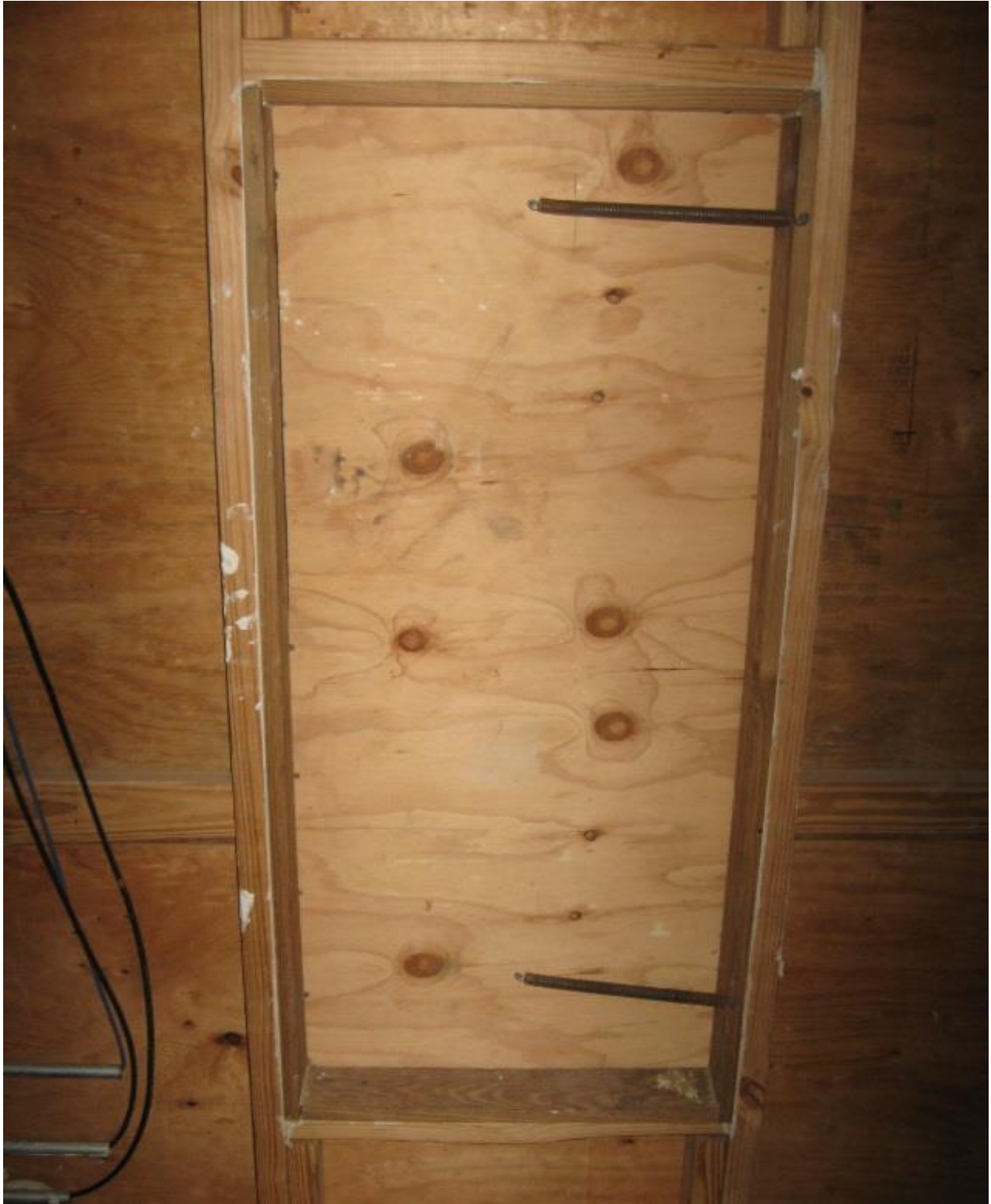
Picture 03 – Typical Door in Plywood Draftstopping
