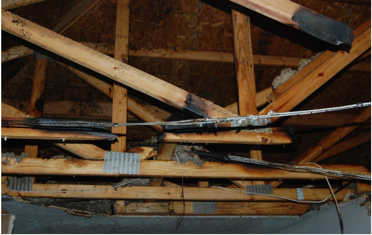
Picture 18 – Lightning Strike in Wood Attic.
