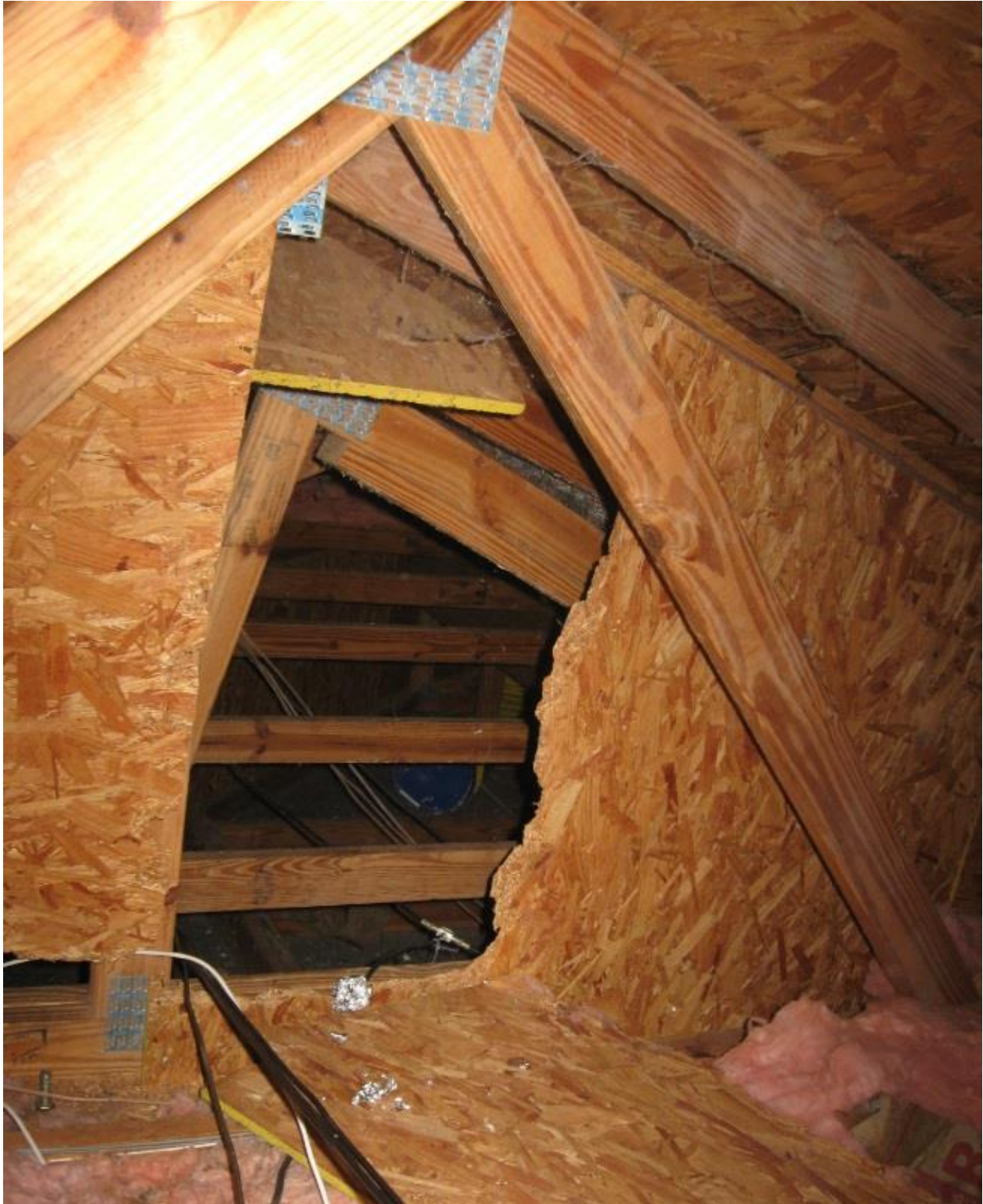
Picture 13 – Building 15 Deficiency.
