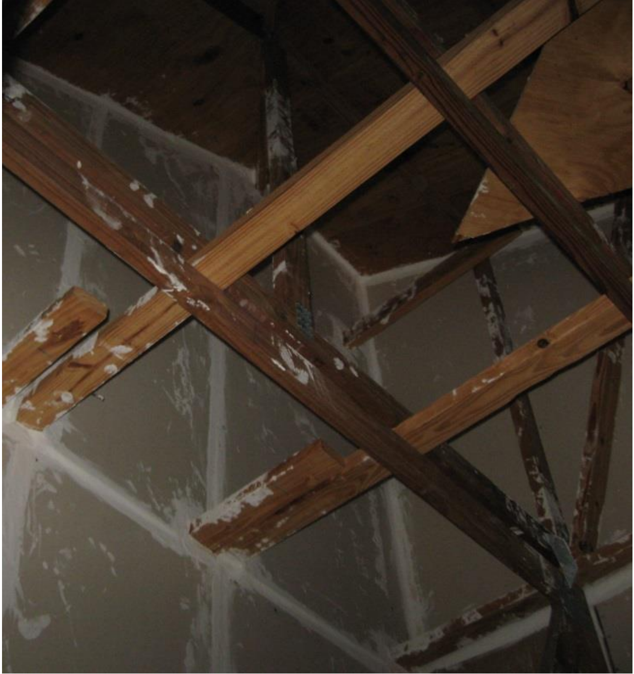
Picture 05 – Gypsum Draftstopping with All Penetrations and Joints Sealed with Mud and Tape
