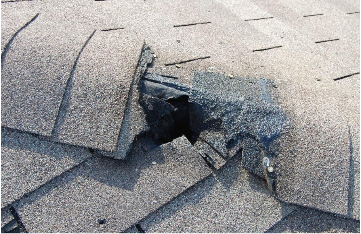
Picture 17 – Lightning Strike through Roof
