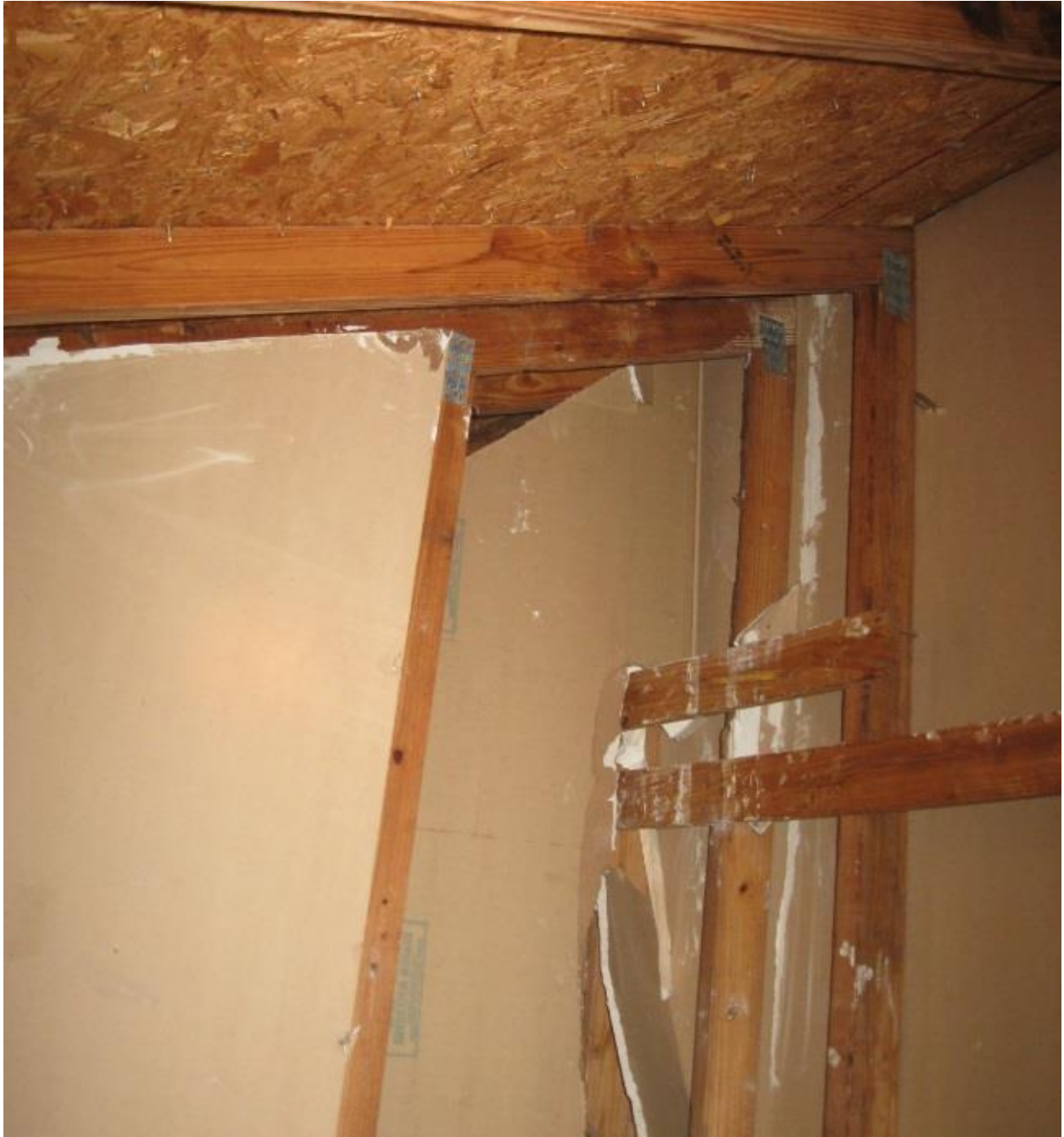
Picture 09 – Building 11 Deficiency.
