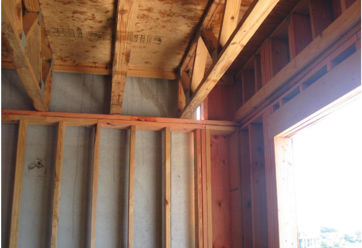
Picture 15 – Floor Terminating into Exterior Walls in Type III Construction with Exterior Walls of Fire-Retardant-Treated Wood at Concrete Fire Wall
