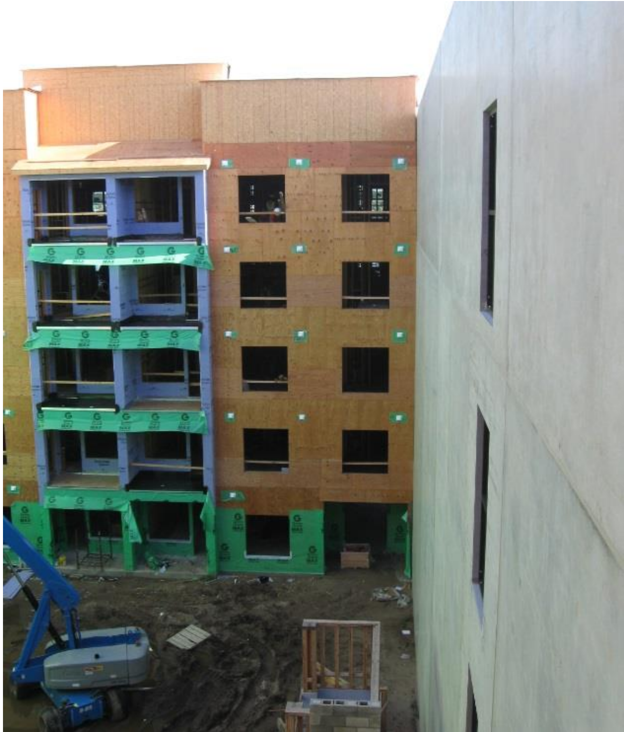
Picture 14 – Type III Construction with Exterior Walls of Fire-Retardant-Treated Wood Adjacent to Concrete Parking Garage
