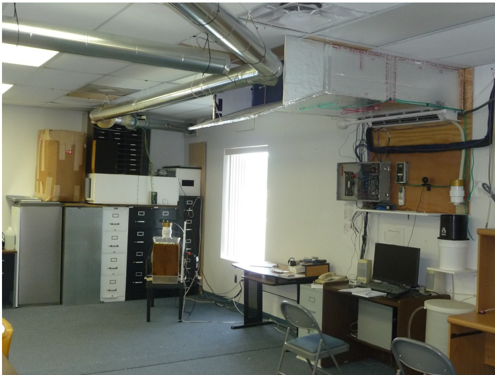
Figure 2. Minisplit with OA duct termination at return intake plenum.
