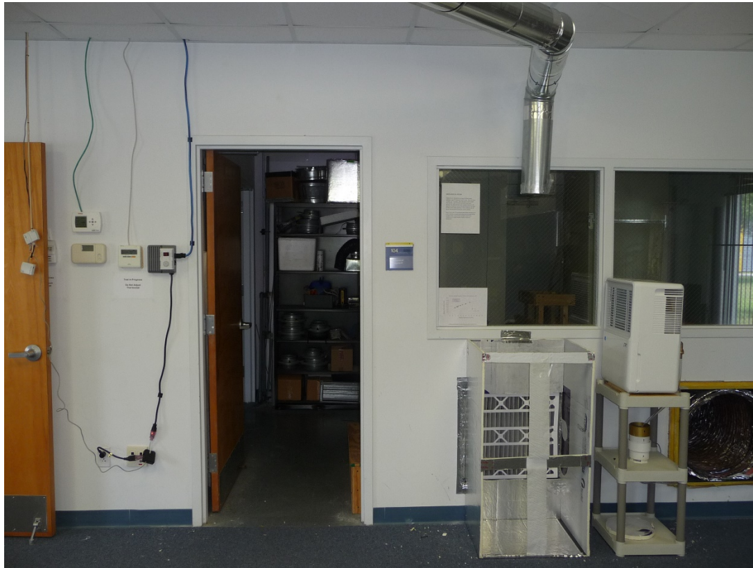
Figure 3. View of thermostat and remote dehumidistat on wall at left and view of OA duct termination just above the central intake return. Dehumidifier is on a stand on the right side.
