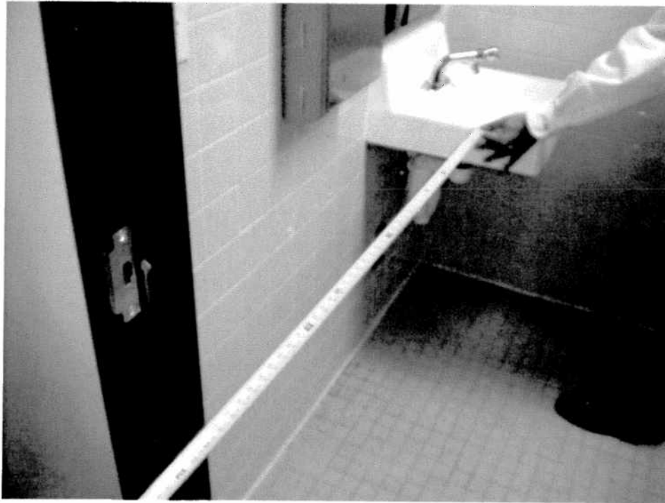
Restroom 201A – Distance from lavatory to doorway is 44”.
