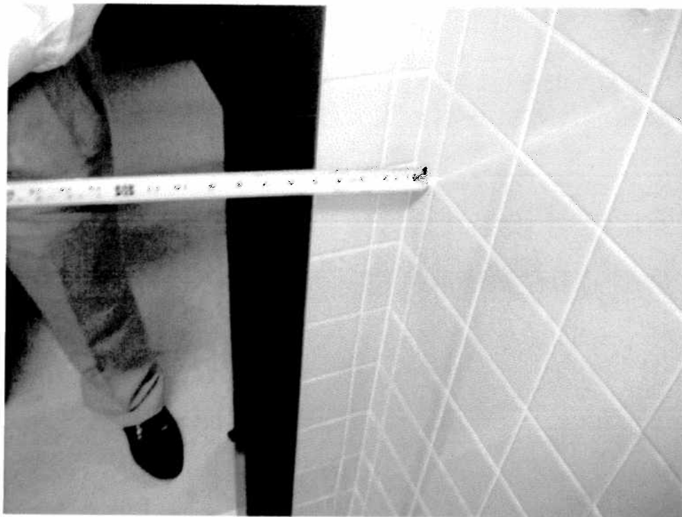
Restroom 201A – Clearance on push side of door is 7”.
